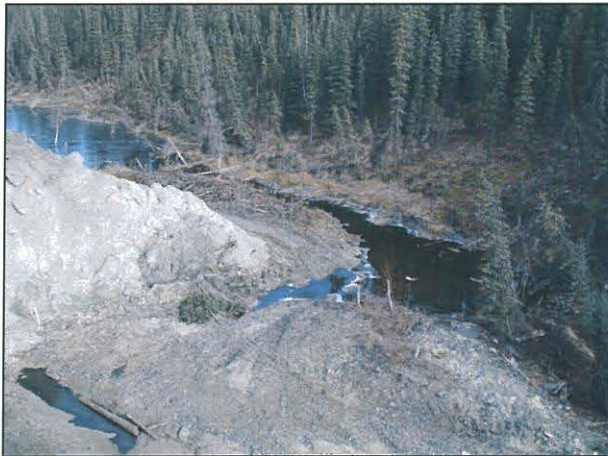
Figure 5.4 Wolverine Creek Channel At Upstream End Of South Lobe After Maintenance Work Completed
