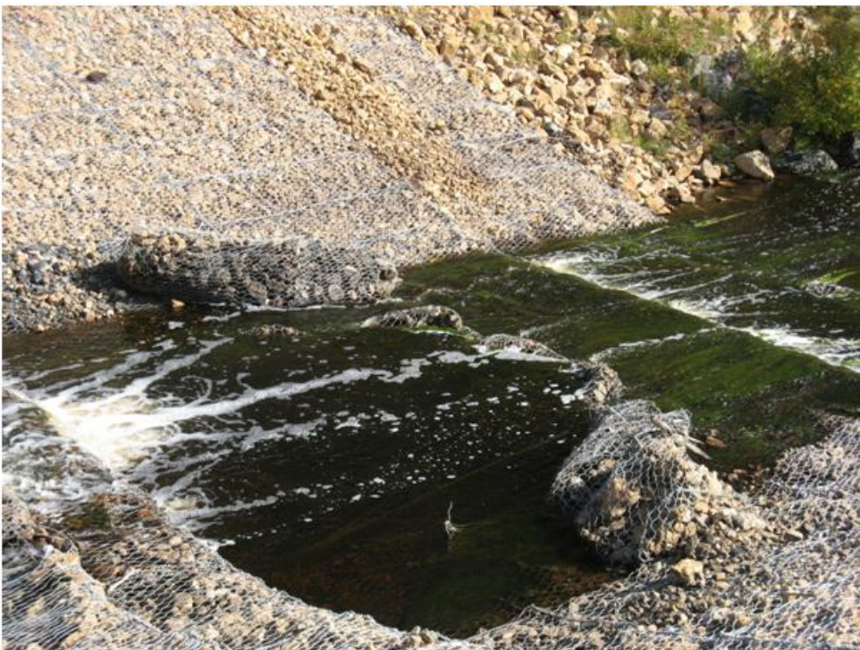
Photo 14: Drop Structure #4 prior to construction. The downstream sill has been damaged.
