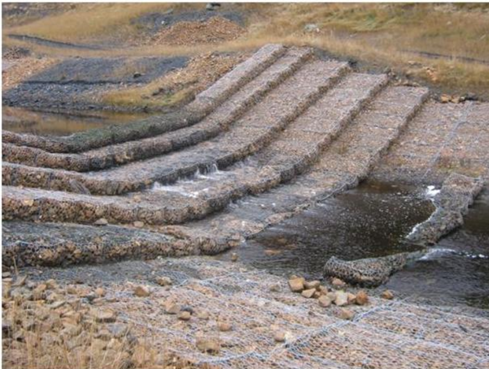
Photo 12: Drop Structure #3. All compartments have been filled with rock and closed. The end sill is deformed a little but is still intact and attached to the gabions below.
