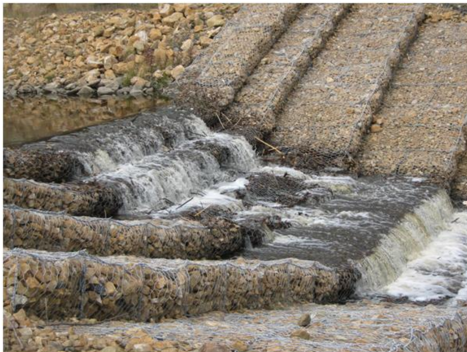
Photo 5: Drop Structure #2 prior to construction. Gabion compartments are open and partially full to empty.
