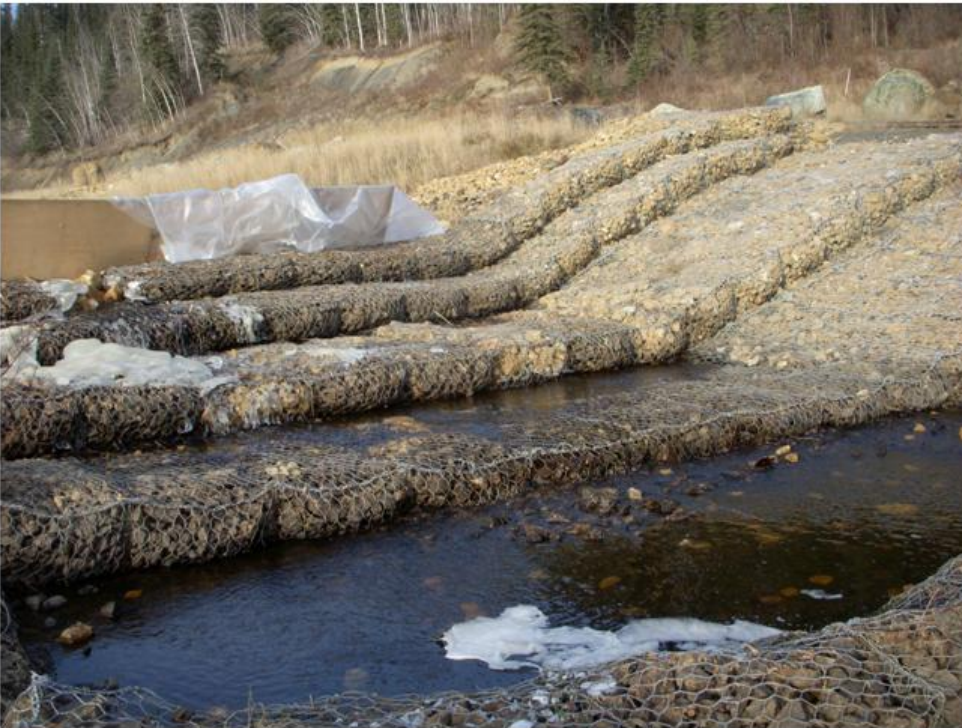
Photo 2: Drop Structure #1, looking upstream. All compartments have been filled with rock and closed. Flow in Creek partially blocked using plywood and plastic sheets.
