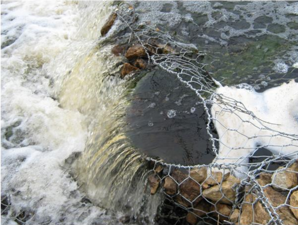
Photo 11: Drop Structure #3 prior to construction. The downstream top edge of a gabion basket as come open.
