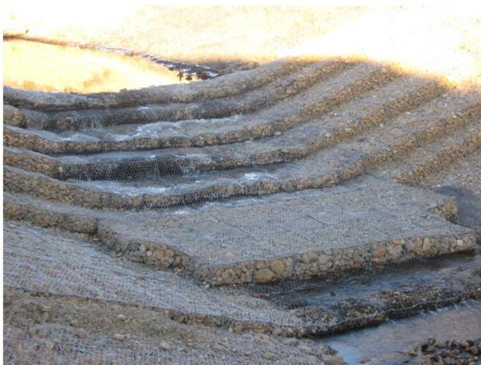
Photo 21: Drop Structure #4. Construction complete including the installation of new 0.5 m gabion baskets at the downstream end of the structure.
