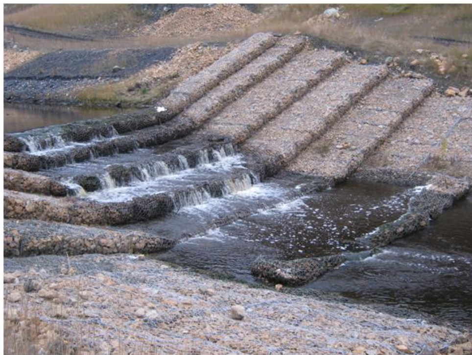
Photo 10: Drop Structure #3 prior to construction. A hole on the top of a gabion basket can be seen on the far back midway up the structure. Some basket repair and some gabion fill is required.
