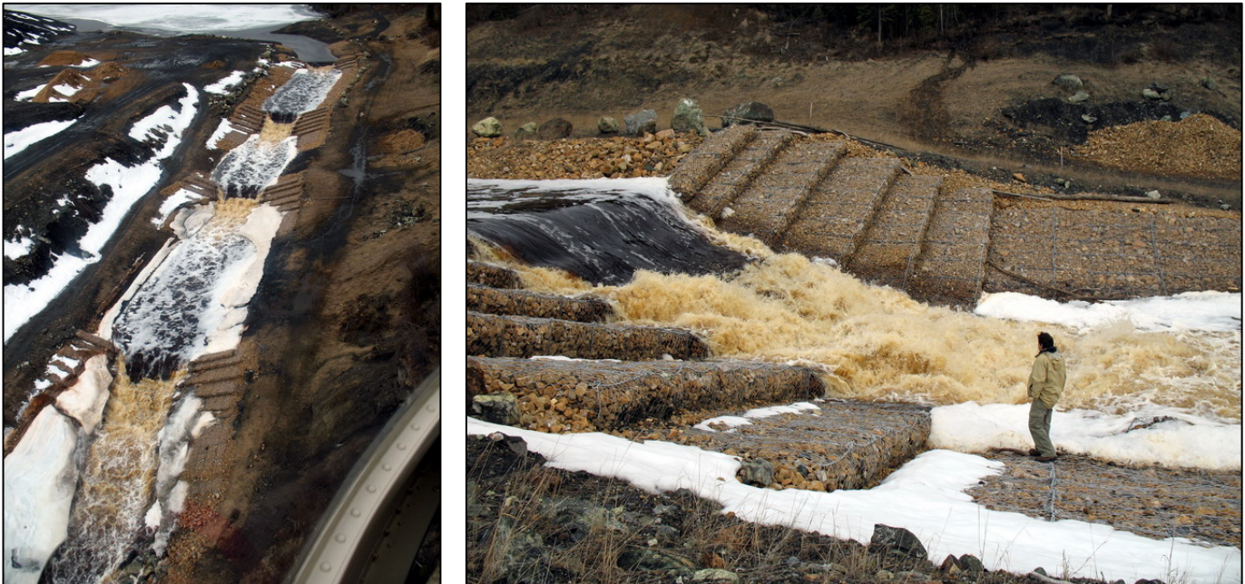
Figure 2: Gabion Drop Structures in May 2009 (DS#2 on Right Hand Side of Photo)
