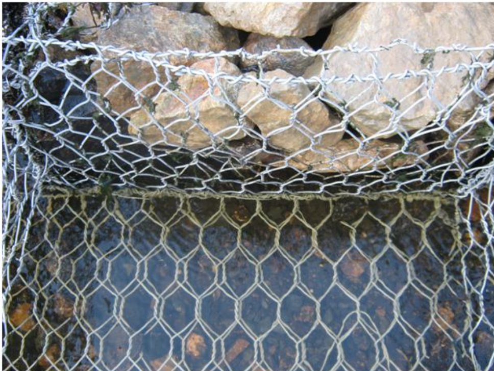
Photo 18: Drop Structure #4. The upstream bottom end of the new 0.5 m baskets were hand stitched to the existing structure.
