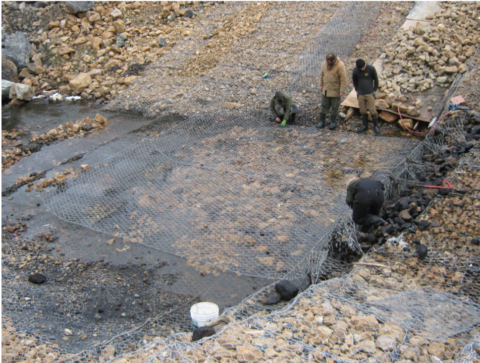
Photo 17: Drop Structure #4. Placement of the mat at the location of the filled hole, downstream end of the structure.
