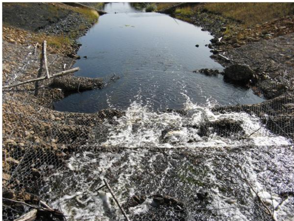
Photo 6: Drop Structure #2 prior to construction. Middle section of the downstream sill has been damaged.
