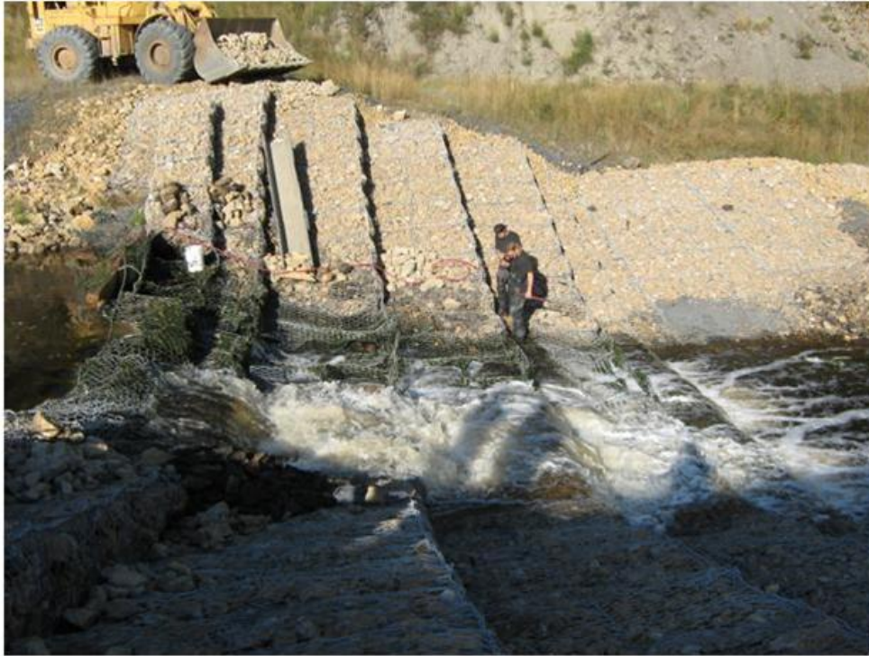
Photo 15: Drop Structure #4. Empty baskets within the structure.
