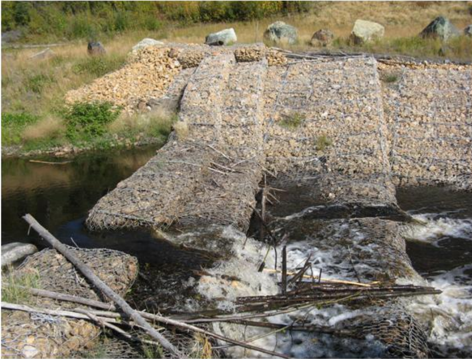
Photo 1: Drop Structure #1, looking to the left bank prior to construction. Debris has accumulated in the drop structure and one gabion compartment is open along the downstream top edge.
