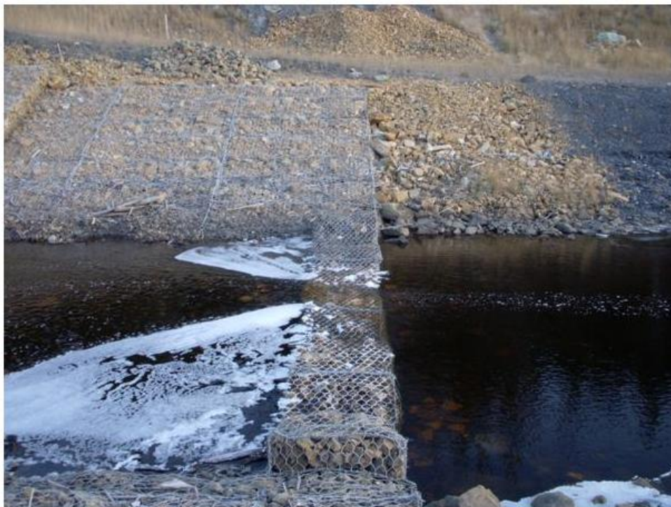
Photo 8: Drop Structure #2. New 0.3 m end sill placed at the downstream end of the structure.
