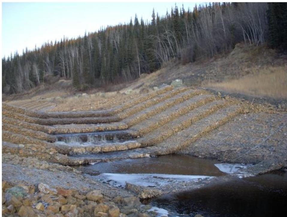
Photo 7: Drop Structure #2. All compartments have been filled with rock and closed. The new end sill has been placed at the downstream end of the structure.
