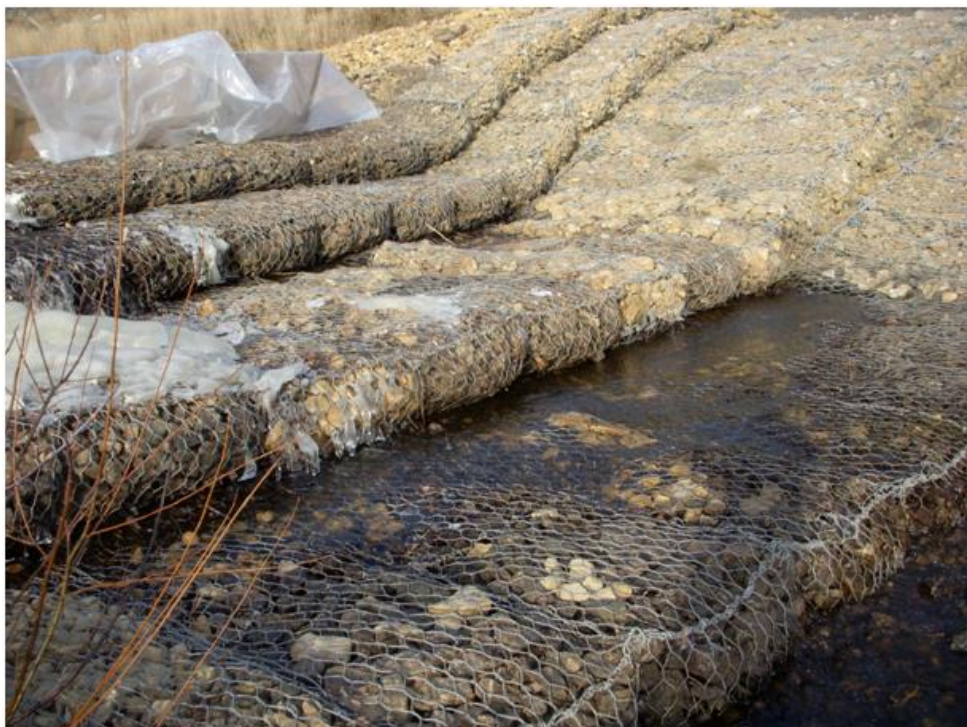
Photo 3: Drop Structure #1, looking upstream to left bank. All compartments have been filled with rock and closed.
