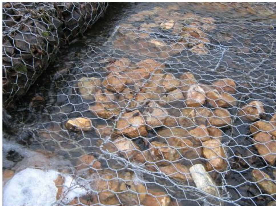
Photo 4: Drop Structure #1. New gabion tops hand stitched on the upstream and downstream edges.
