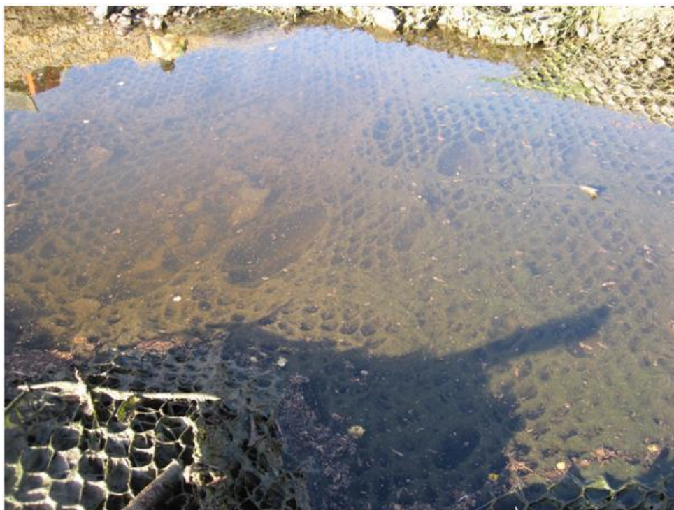
Photo 4. Drop Structure #3. Partially empty gabions and damaged wire mesh at the structure floor.
