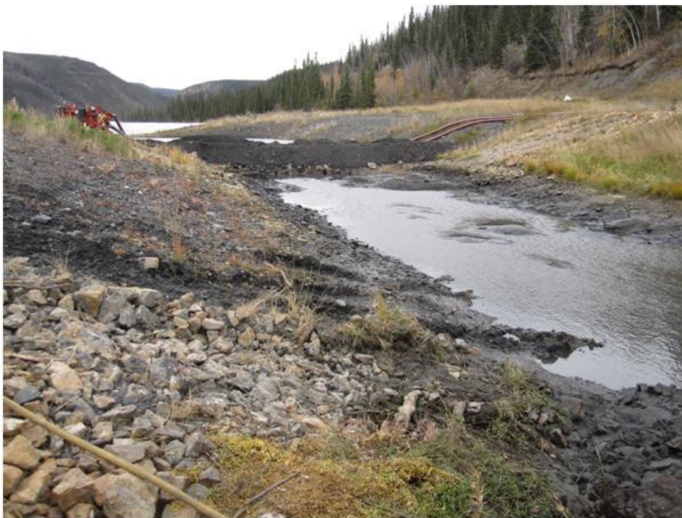
Photo 10. Second coffer dam located upstream of Drop Structure #1, looking upstream. The second coffer dam was placed after the first dam was removed to allow work on Drop Structure #1 and the downstream channel between structures #1 and #2.
