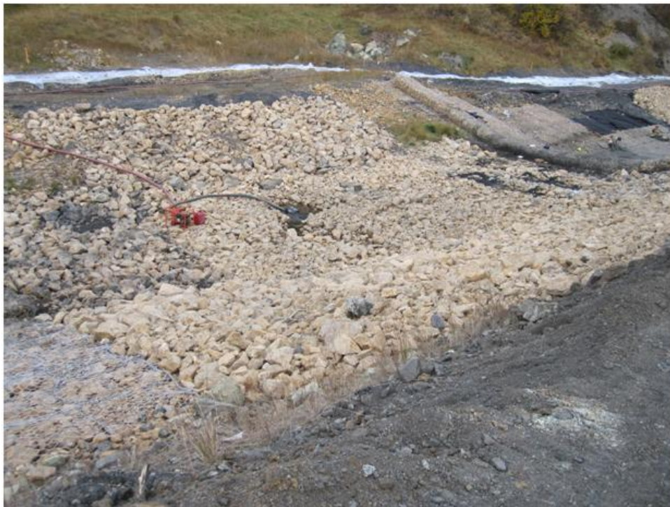
Photo 17. Channel side slopes reshaped and fill material placed to the original design elevation within the channel bottom between drop structures #2 and #3.
