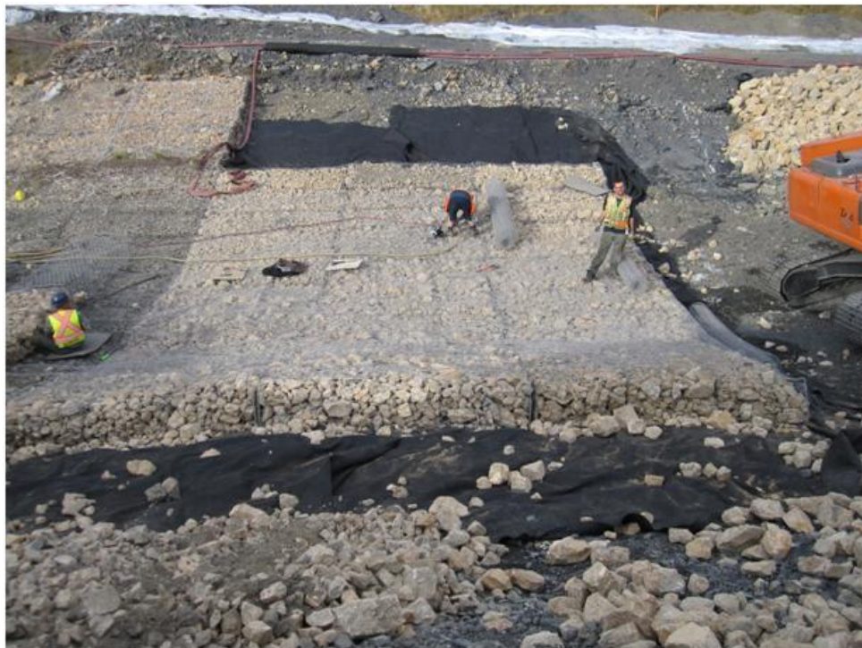
Photo 15. Gabion baskets being filled with rock at the downstream end of Drop Structure #3. New gabion end sill being filled with rock at the left side of the picture.
