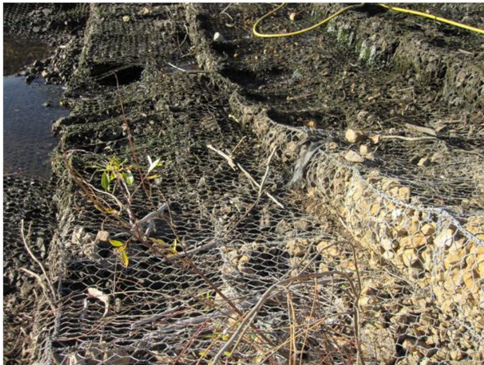
Photo 3. Drop Structure #3, looking to right bank. Partially empty compartments and damaged wire mesh prior to construction.
