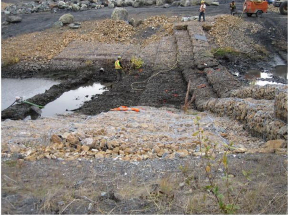
Photo 1. Drop Structure #1, looking to the right bank as construction begins. Minor Rock fill and repair to the gabion mesh at the drops and floor required.
