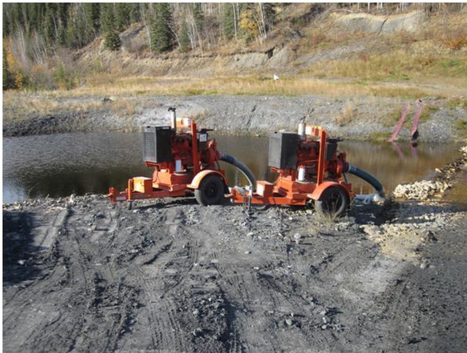
Photo 11. Pumps used when the second cofferdam was in place and discharge through the diversion channel was cut off.
