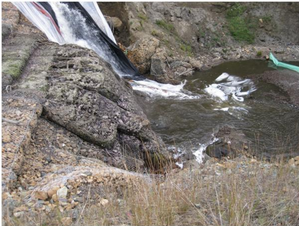
Photo 5. Drop Structure #4 looking to the left bank. The right channel bank had slumped in. No construction occurred at Drop Structure #4
