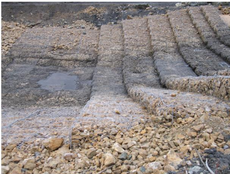
Photo 14. Gabion baskets refilled with rock and mesh material repaired at Drop Structure #2
