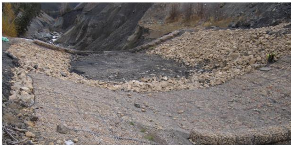
Photo 18. Channel side slopes reshaped with rock rip rap and channel bottom excavated to original design elevation. A Three metre wide rip rap section placed adjacent the downstream end of Drop Structure #3.
