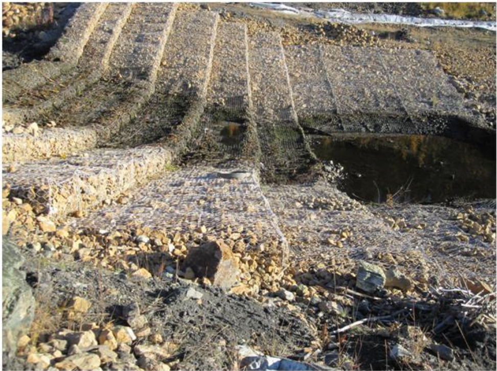
Photo 2. Drop Structure #2, looking to the left bank before construction. Gabions within the steps and at the floor require rock fill and patching of the wire mesh.
