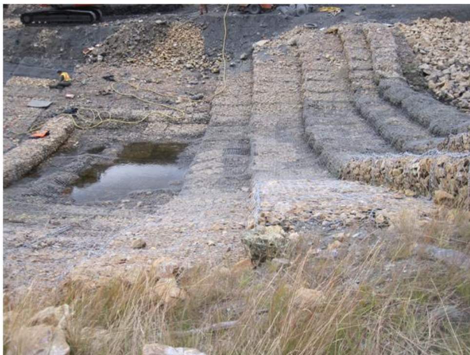
Photo 16. Gabion baskets refilled and gabion mesh repaired at Drop Structure #3. Gabion wire mesh rolled overtop of the existing gabion baskets and secured with C-rings.
