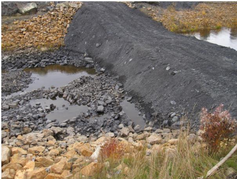
Photo 9. First coffer dam located between drop structures #1 and #2, looking towards the right bank.
