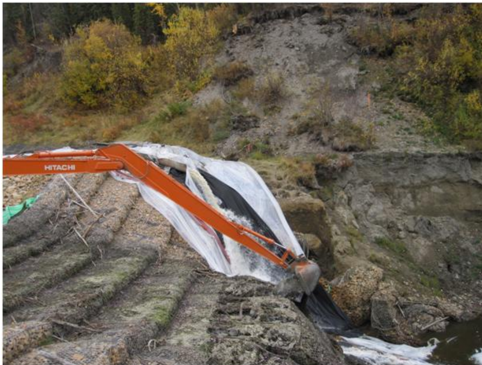
Photo 13. 200 Hitachi Excavator placing boulder material at the downstream end of Drop Structure #4. Other than two test boulders, no material was placed at the downstream end of Structure #4.
