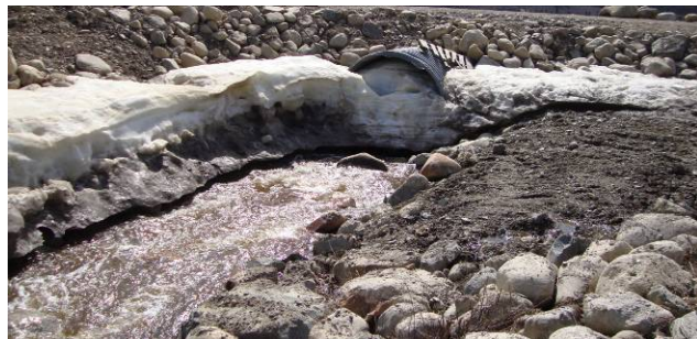
Photo 9: Blocked culvert at downstream end of NWID.
