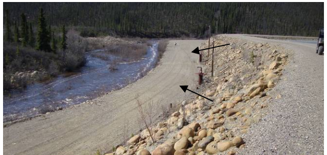
Photo 10: Tension crack along lower bench upstream of the tailings facility near start of RCDC.
