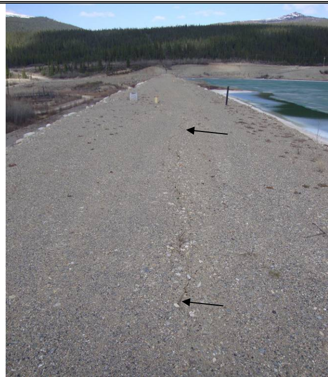
Photo 17: CVD longitudinal tension cracks on dam crest.
