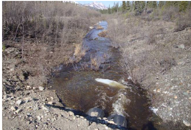
Photo 7: Blocked culvert discharge at service road crossing looking downstream along NWID.
