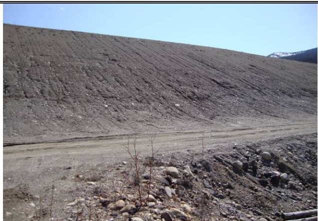
Photo 18: ID downstream slope erosion conditions.
