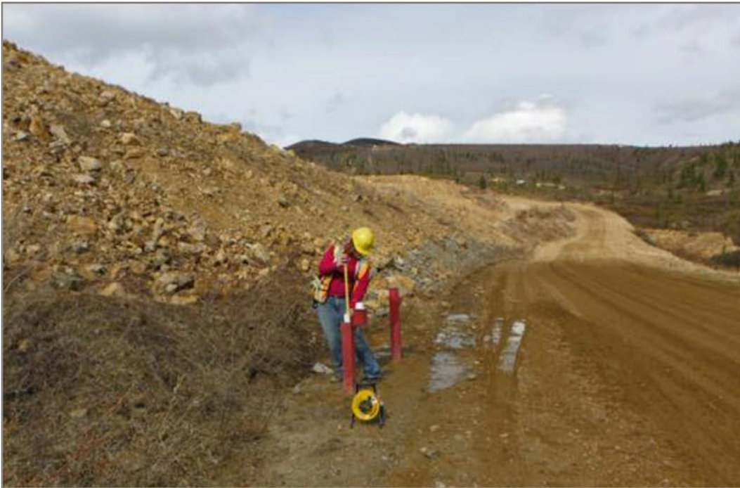
Photo 6: MW09-13 and MW09-14 along the Main Mount Nansen Access Road East of the Open Pit. June 4, 2012
