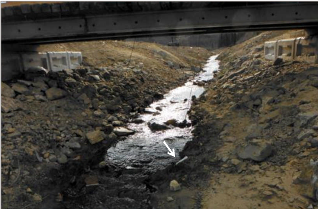
Photo 22: MP09-06 Located under the Dome Creek Diversion Ditch Bridge (indicated by arrow). Note that the mini-piezometer is destroyed. June 4, 2012
