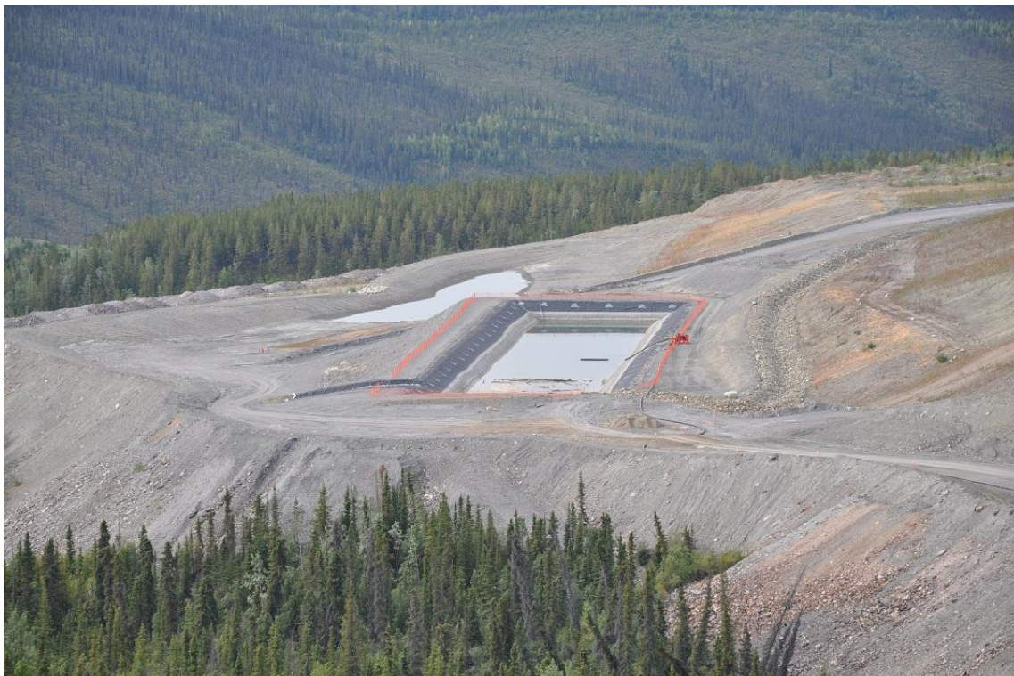
Photo 2-1. View of the rectangular lined pond in the mid-ground and the unlined pond in the background at the toe of the GSC cover (Aug. 22, 2012).
