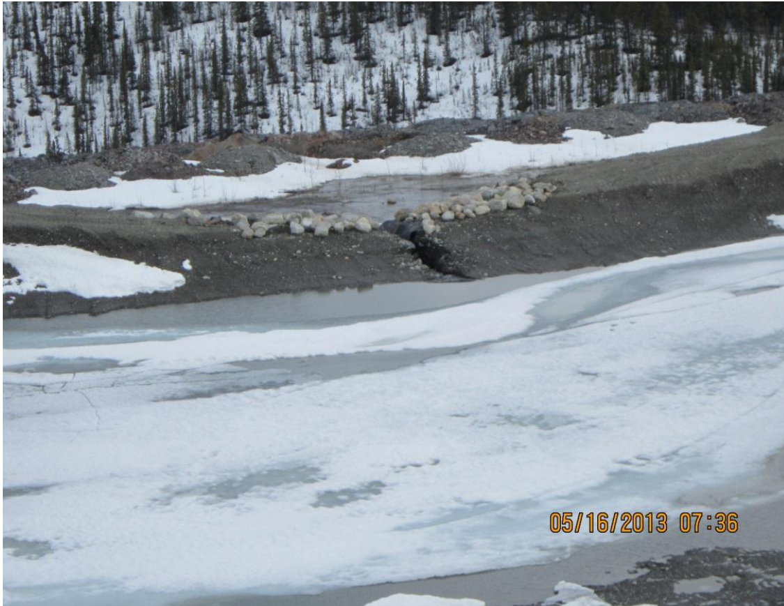
Photo 2-3. View of the breach on the unlined pond berm (May 16, 2013).
