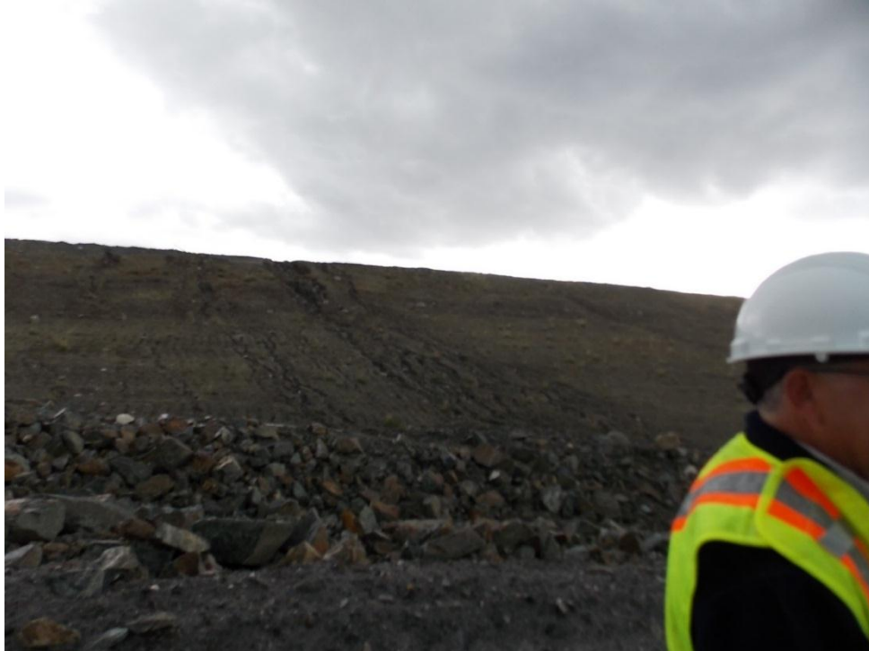
Photo 3-7. Gullies on the toe berm slope (June 13, 2013).
