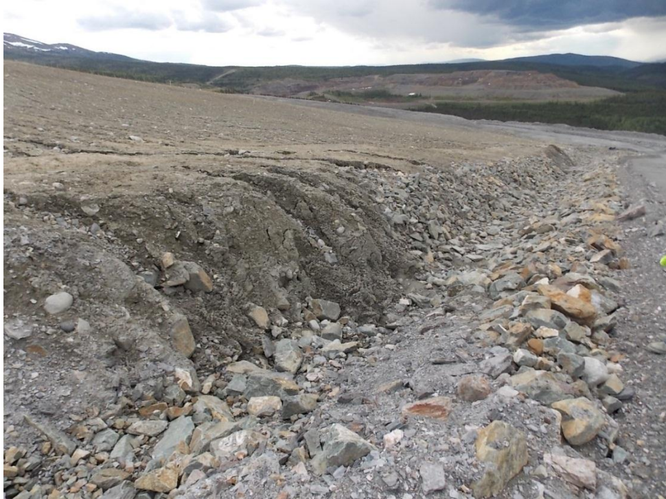
Photo 3-6. Gullies and local cover slough on the inside of the south perimeter ditch (June 13, 2013).
