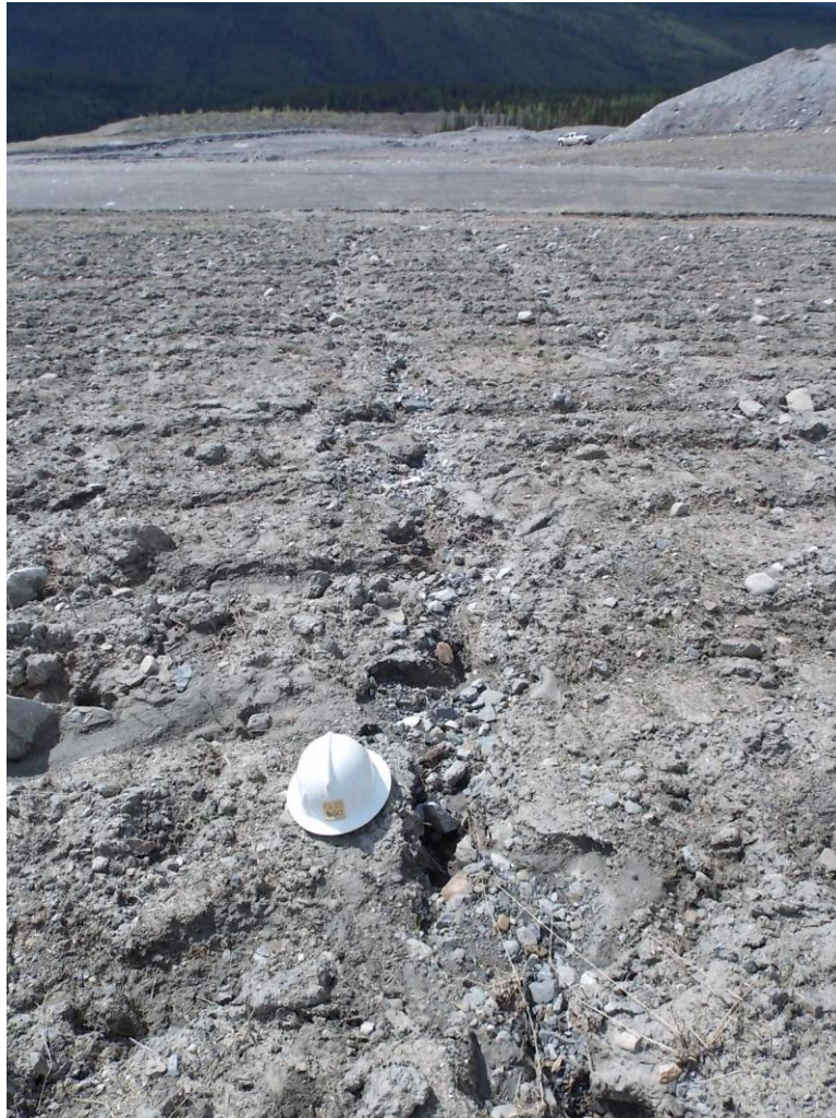
Photo 3-5. Transverse gully on cover surface (June 13, 2013).
