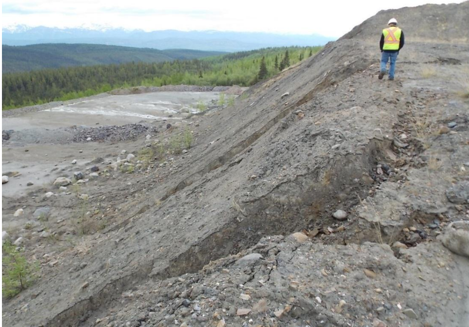
Photo 3-8. Deep incised gully on the toe of the dump face (June 13, 2013).
