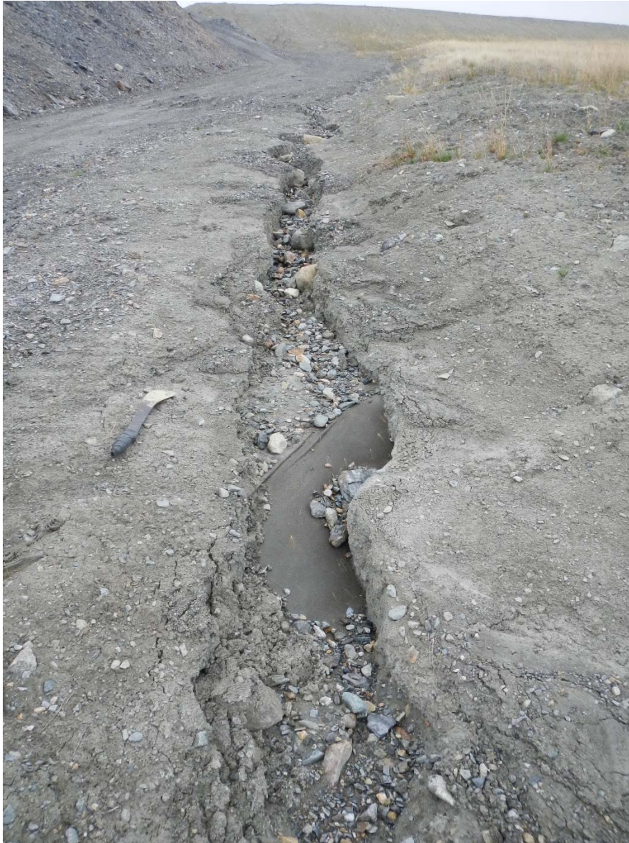
Photo 3-11. Underlying geotextile exposed in West Access Ramp (May 27, 2015) which should be repaired.
