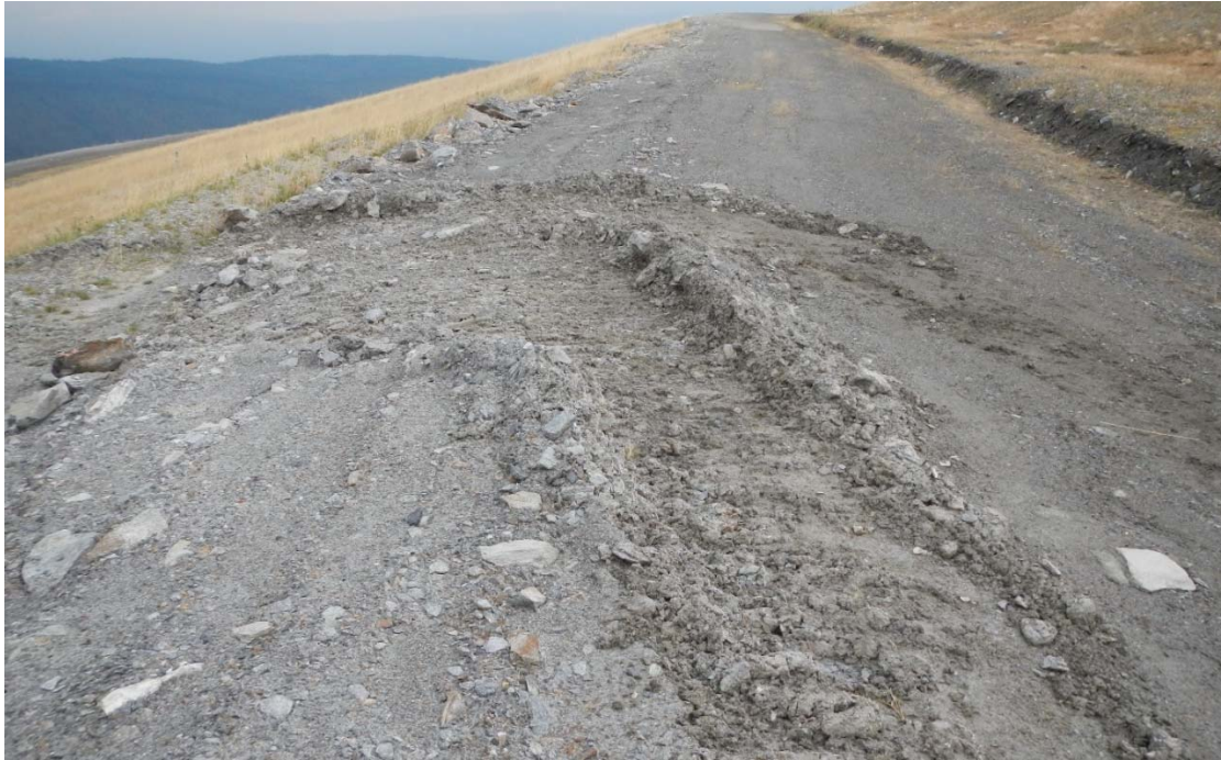
Photo 3-5. View of the excavator tracks and resultant bench disturbance on third bench and then heading left in downhill direction (May 27, 2015). This disturbance will interrupt surface water flow and lead to erosion in select locations.
