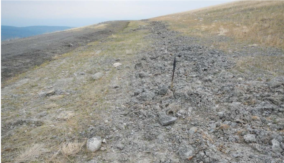
Photo 3-7. View of loose ditch cleaning debris placed on vegetated slope above fourth bench; loose material may erode easily in the future (May 27, 2015).
