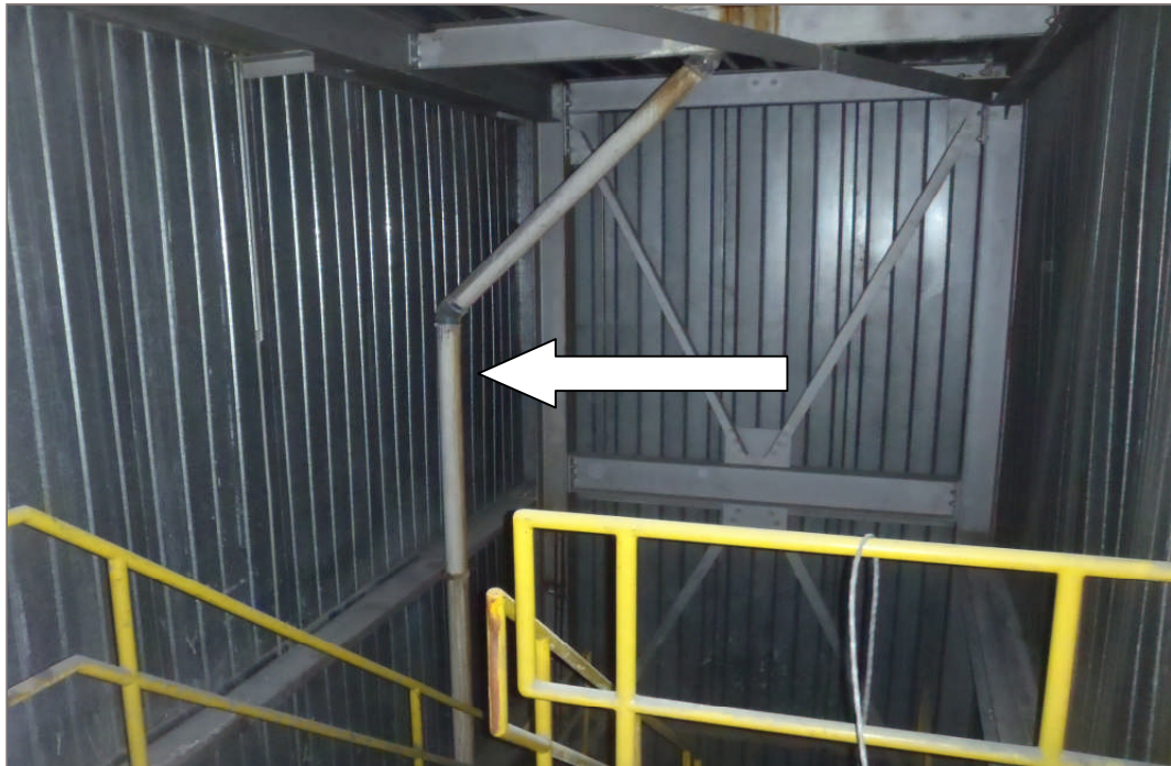
Photo 18: Asbestos containing transite rain water leader's located in a western stairwell off the office area of the Mill.
