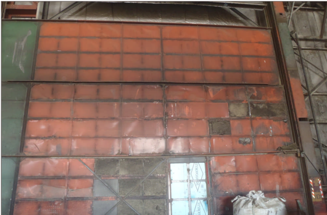
Photo 20: Red lead based paint requiring regulated disposal applied to the overhead doors of the Warehouse.
