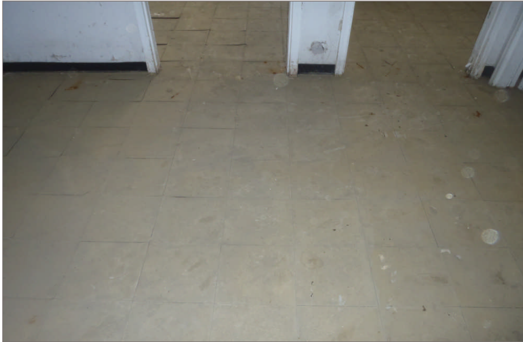
Photo 11: Asbestos containing 12"x12" beige vinyl floor tile located throughout the second floor of the Warehouse and main floor office off the lab.
