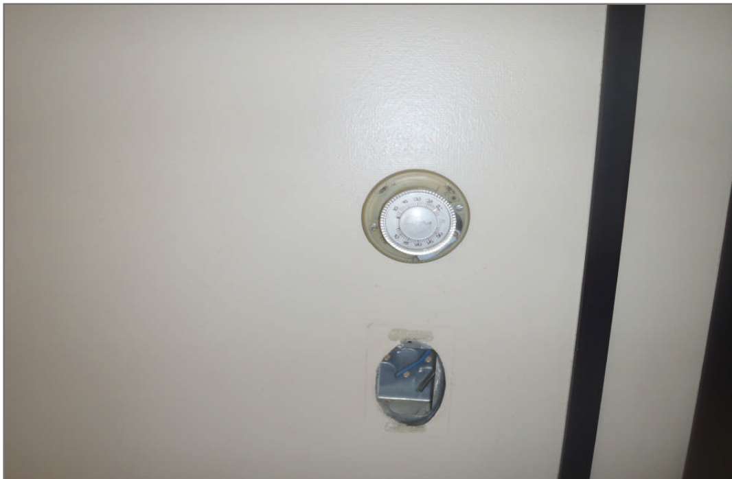
Photo 26: Wall mounted mercury containing thermostat.
