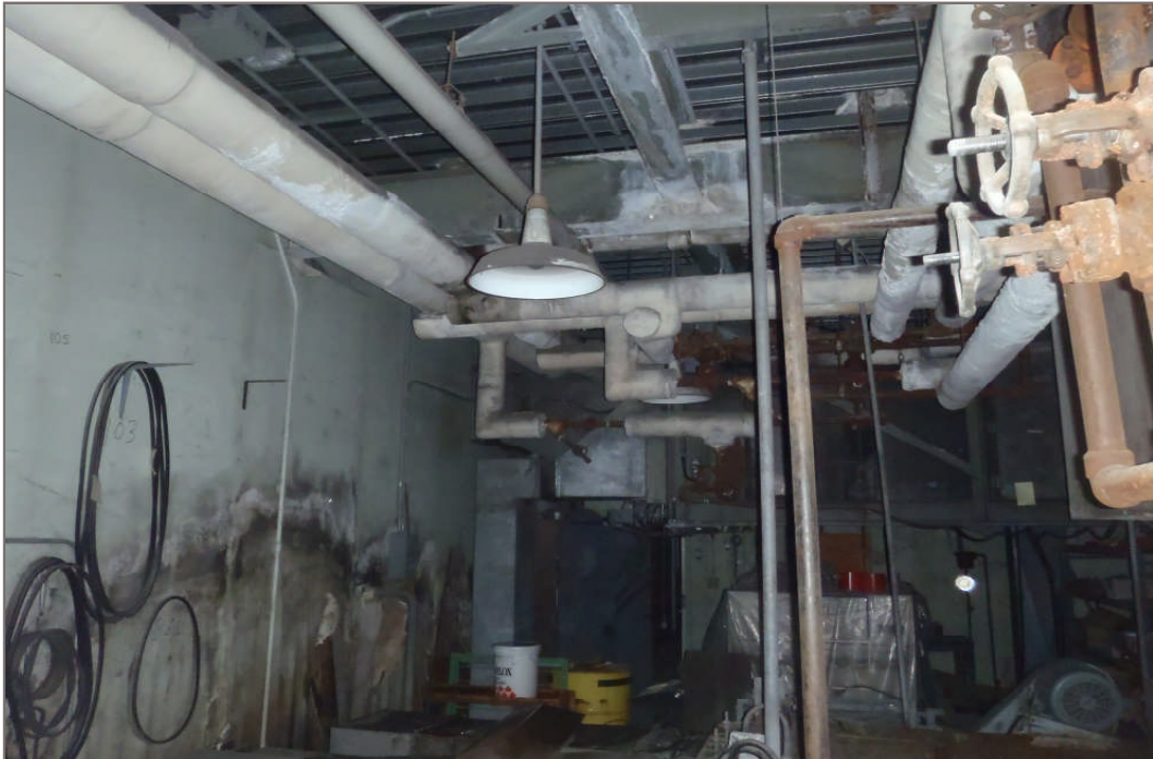
Photo 9: Mould impacted drywall and asbestos containing pipe insulation within the 2 nd floor boiler room of the Warehouse
