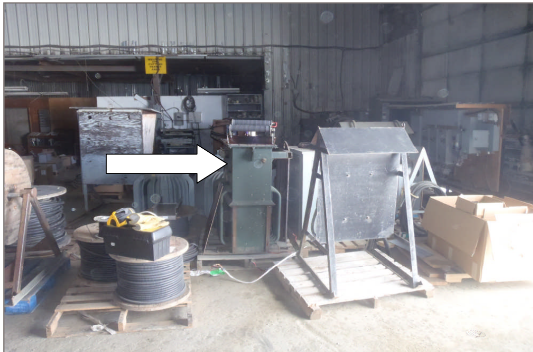
Photo 24: Transformer 25741 sampled for PCB content in cooling oil. Additional transformers in storage were listed as not containing insulating oil.
