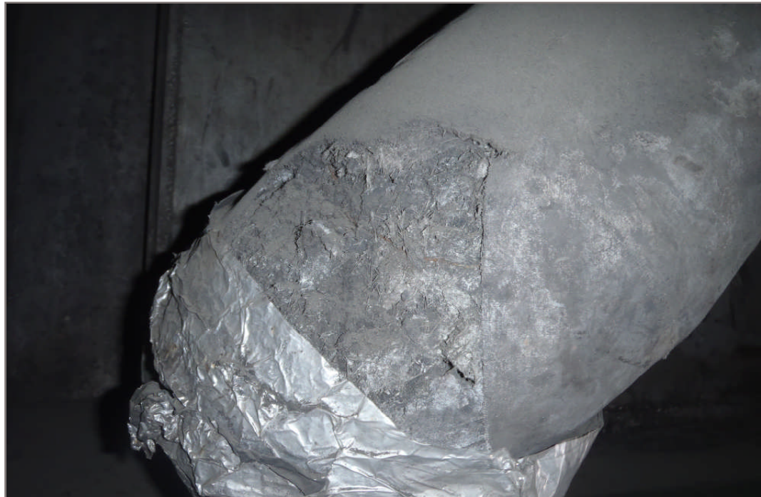
Photo 14: Asbestos containing pipe insulation within the Mill
