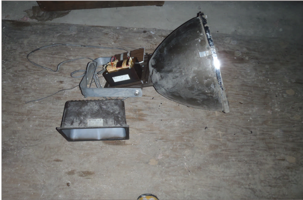
Photo 23: Ceiling mounted high pressure sodium light housing a PCB-containing light ballast.
