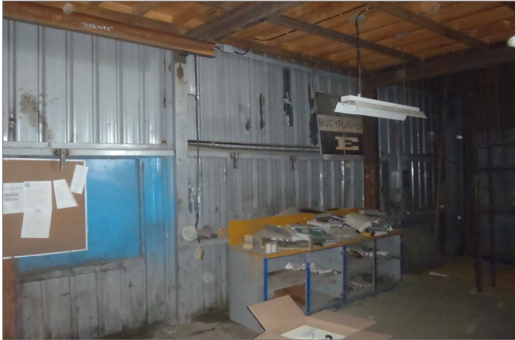
Photo 21: Grey lead based paint requiring regulated disposal located in the welding shop of the Warehouse.
