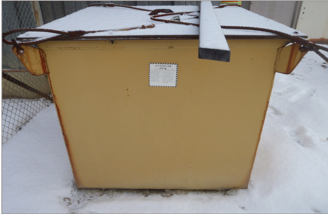
Photo 25: Transformers adjacent to the electrical yard behind the Mill stating PCB containing insulated oil.
