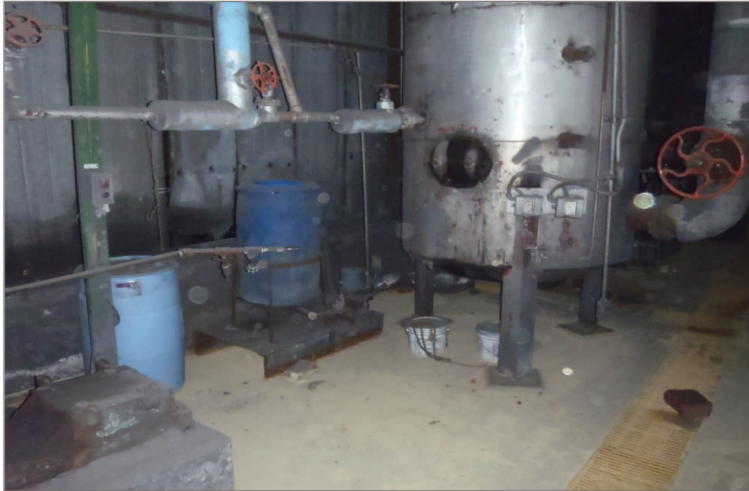
Photo 15: Asbestos containing pipe insulation associated with a boiler in the mill
