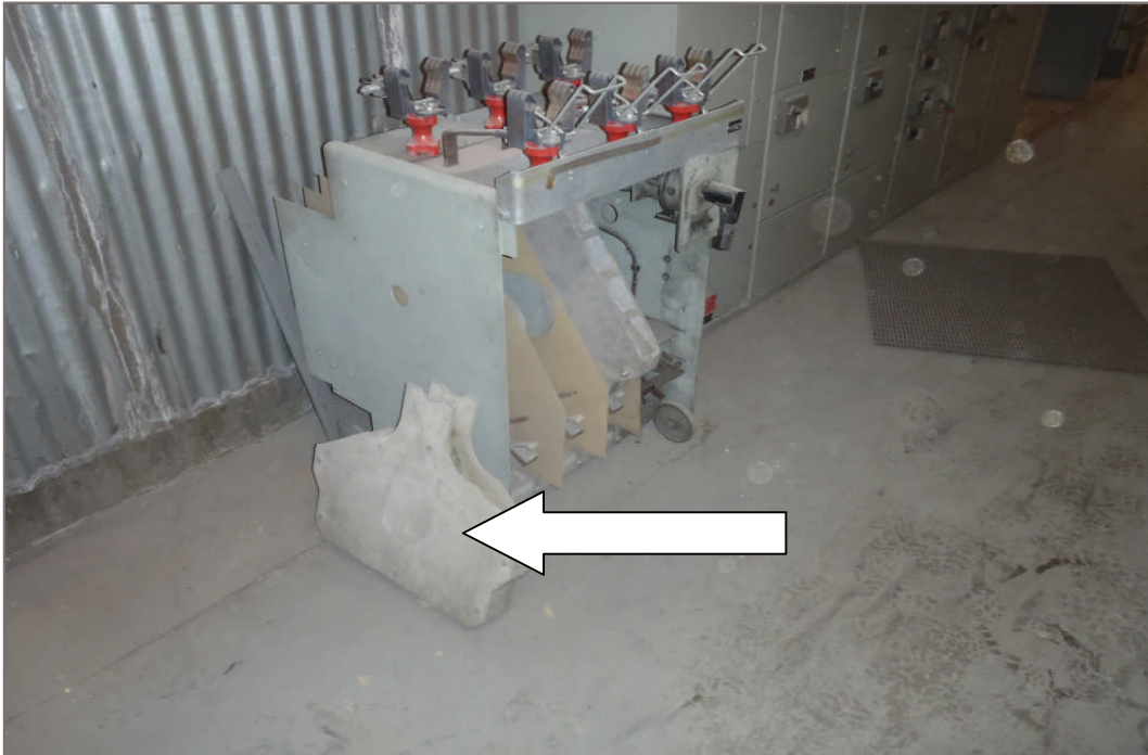
Photo 19: Asbestos containing transite cement board used as electrical components within the Mill
