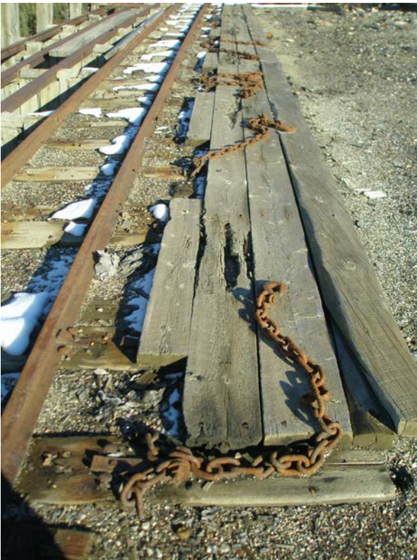
The load out is constructed with log cribbing notched at the corners and consecutively along the width of structure, and sheathed with rough 2x6.
