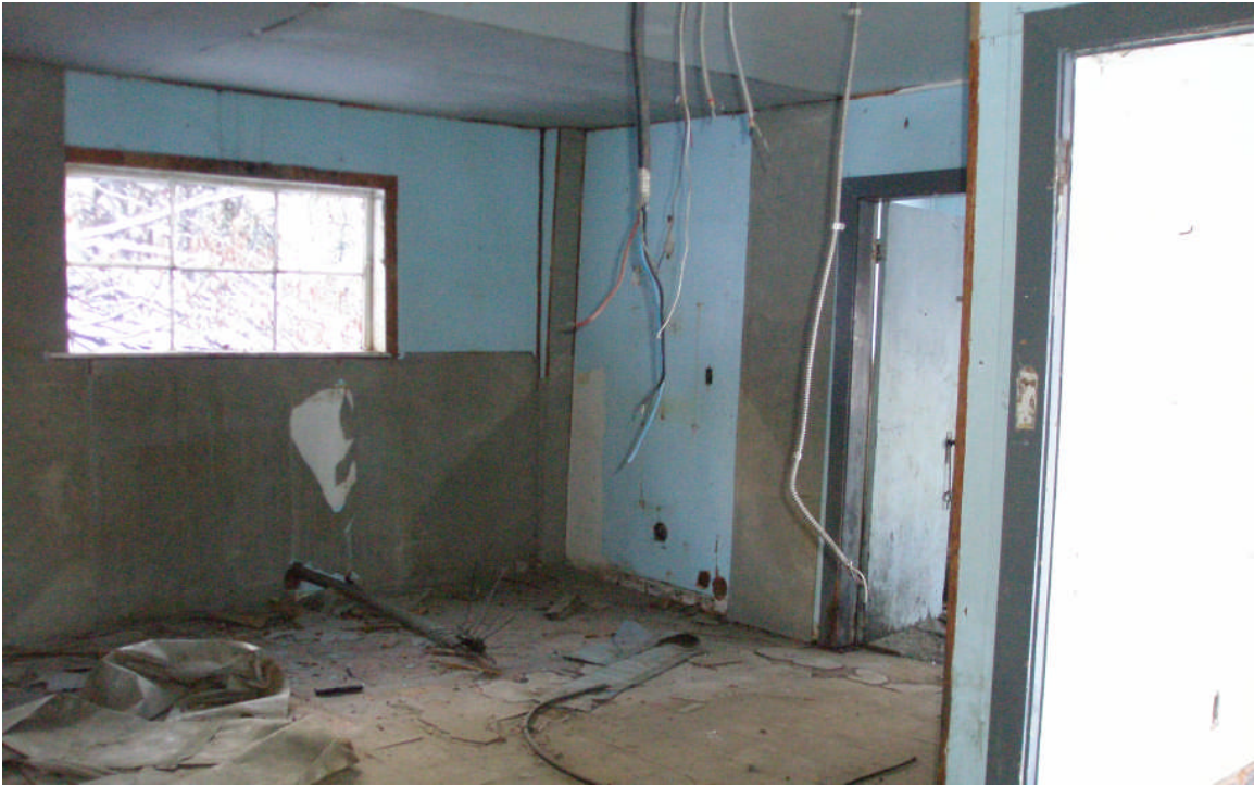
The middle section of the building was used as a shifters office and an electrical room as heavy power cable remains along the south wall and asbestos sheets are present.
