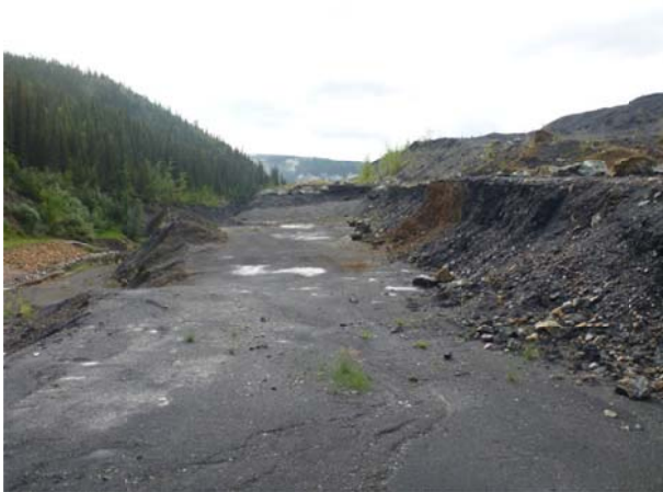
Photo 6 – Road blockage along creek near gabion baskets
