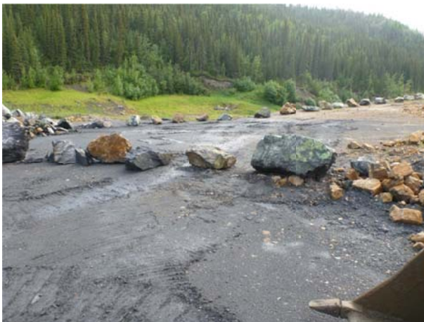
Photo 5 – Road blocked at the gabion baskets to prevent access along creek
