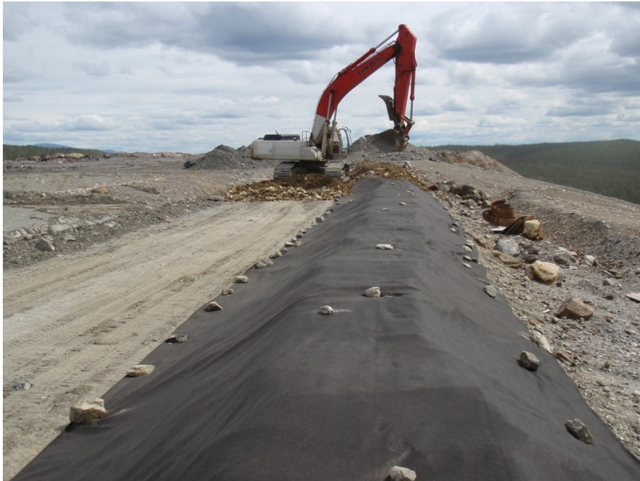
Photo 3: Berm 3 under construction, geotextile overlying compacted till and then clad with rock
