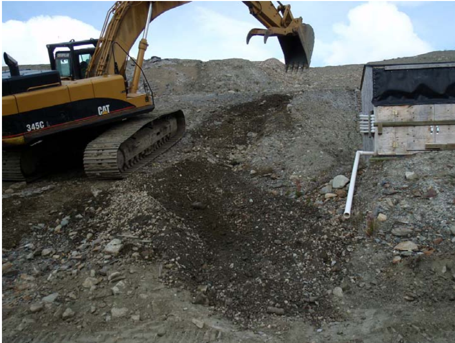
Photo 11: Repairing erosion around the lower monitoring hut by shoring up the gully and placing rock and clean gravel
