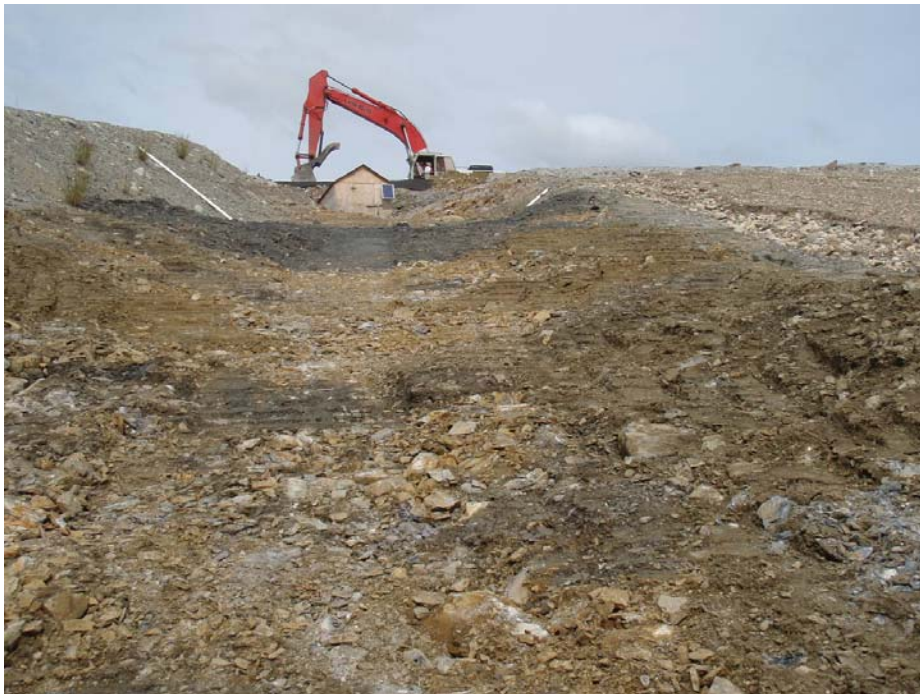
Photo 10: Between CT#4 and CT#3A, erosion repaired, berm repaired and pipelines fixed and covered with soil
