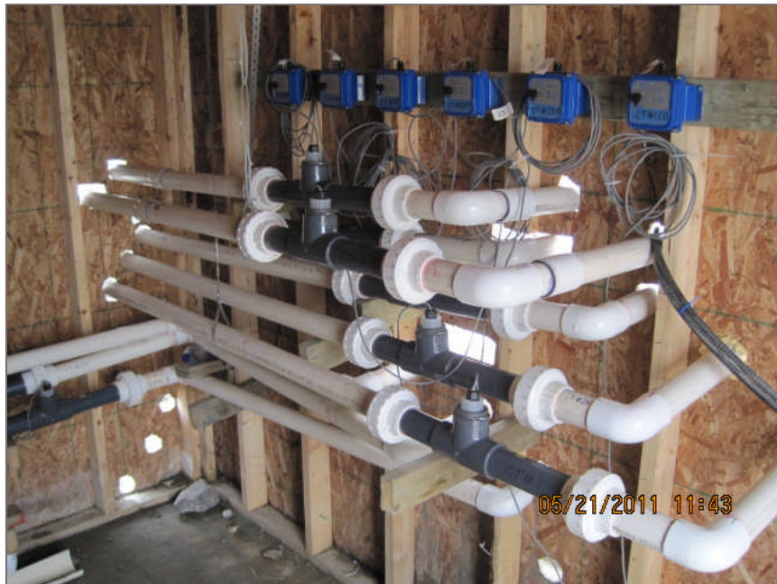
Photo 4: SeaMetric turbine flowmeters and DL75 data loggers installed into the Lower Monitoring hut.
