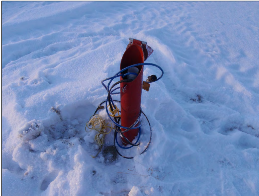
Photo 31: View of well W14103083BH01. Photo taken on February 2, 2016.
