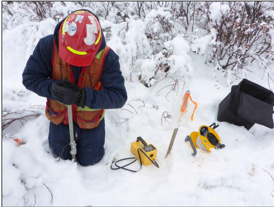
Photo 27: View of drive point wells GSI-PC-04A and GSI-PC-04B. Photo taken on February 3, 2016.
