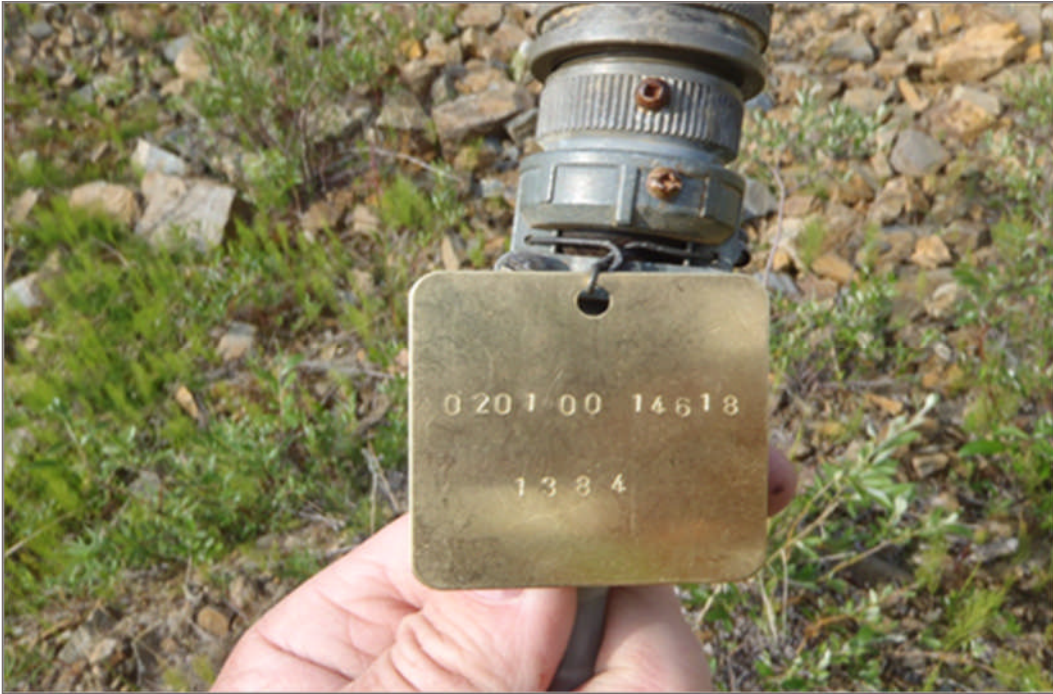
Photo 3: Example of a thermistor cable connector labeled with a brass tag and stamped with the consultant's project number (top) and the individual instrument number (bottom), July 18, 2012
