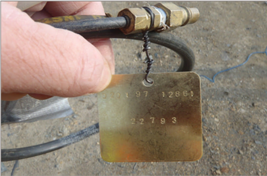
Photo 4: Example of a pneumatic piezometer cable connector labeled with a brass tag and stamped with the consultant's project number (top) and the individual instrument number (bottom), July 18, 2012
