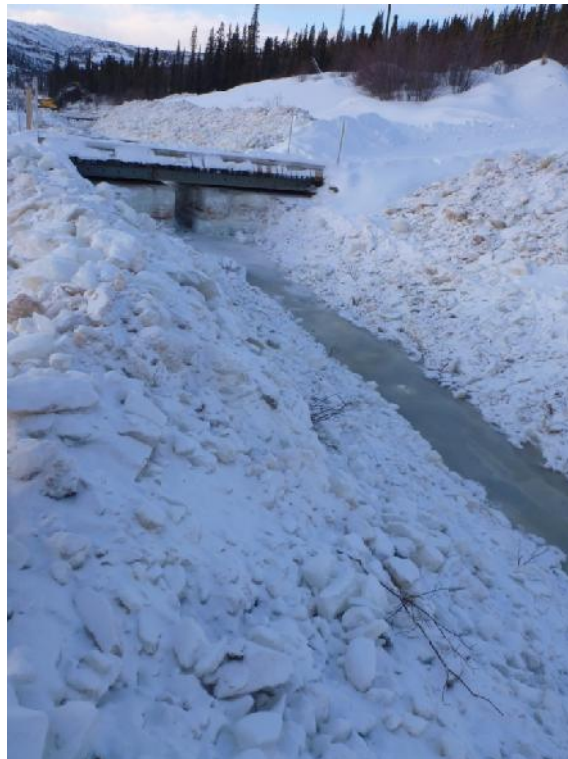
Photo 15. Diversion channel at Bridge (H-DC-B) – Overflow ice conditions on January 9, 2012.
