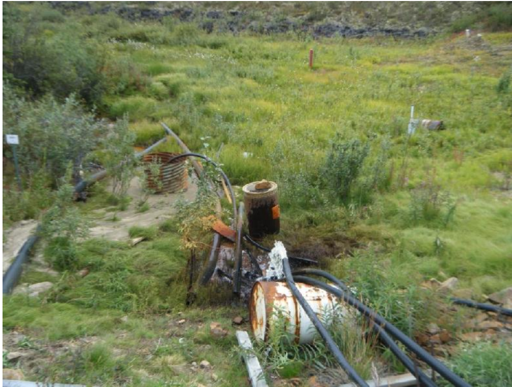
Photo 16. Seepage Site (H-SEEP) - August 18, 2011.
