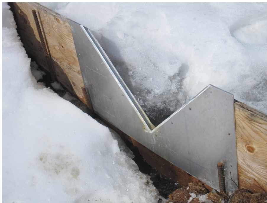
Photo 6. H-PC-U weir showing seepage around weir.
