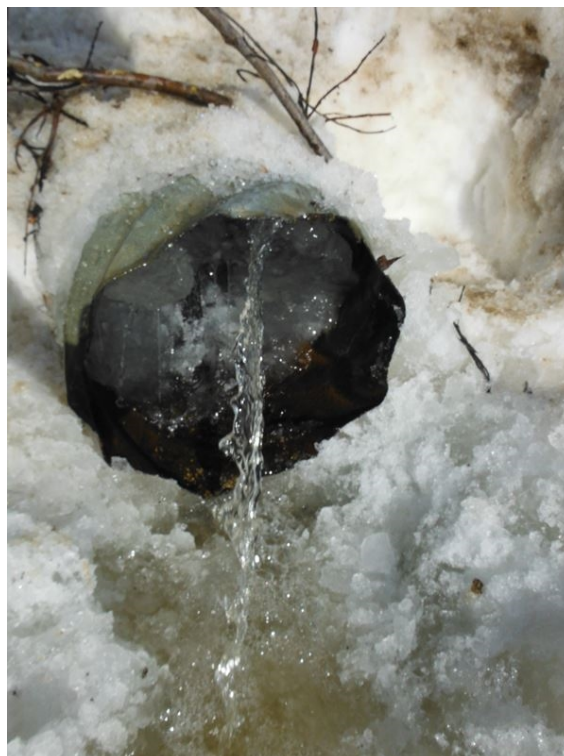
Photo 5. H-PC-DSP culvert ice conditions.
