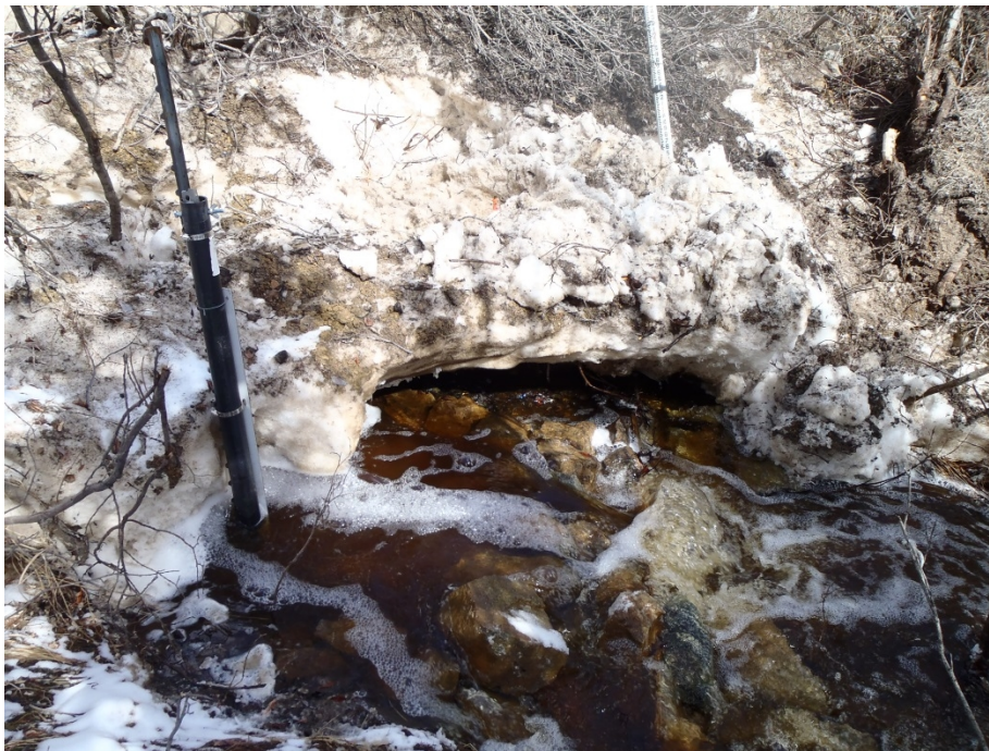
Photo 6. The H-PC-DSP station left bank and stilling well. Snow and ice along ditch below culvert at left. Open water flowing downstream of stilling well.
