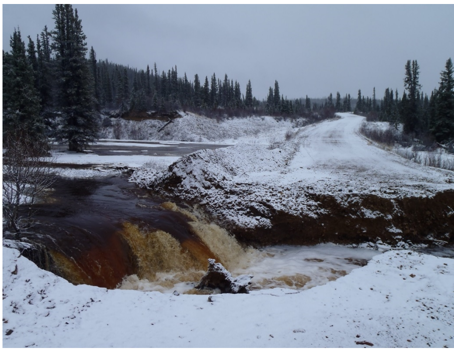
Photo 1. Victoria Creek washout, viewed looking east.
