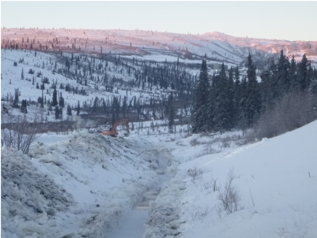
Photo 1. H-DC-B Channel with flow, however excavator activity upstream prevented sampling, December 17, 2013.
