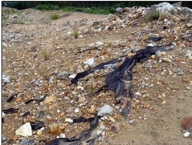
Figure 44 Exposed Geotextile on N Bank at Sta 0+920 (WP 57)
