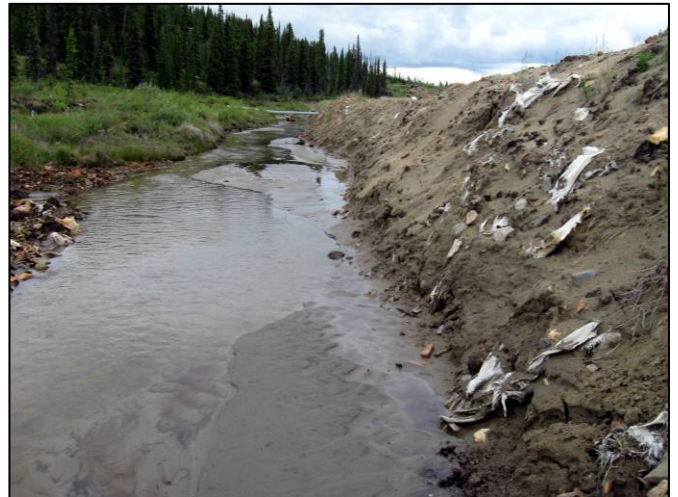
Figure 33 E End of Diversion Channel at Confluence With Dome Creek (View D/S)
