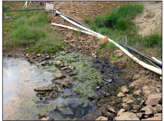
Figure 23 Seepage at NE Corner of Pond
