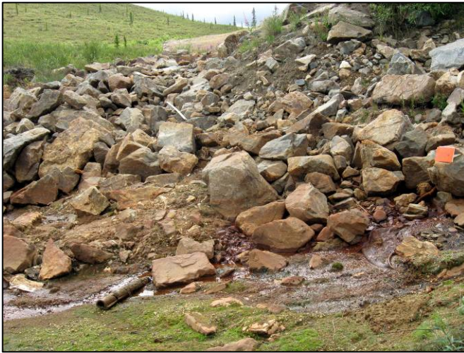
Figure 22 Seepage & Fe Staining at SW Corner of Pond
