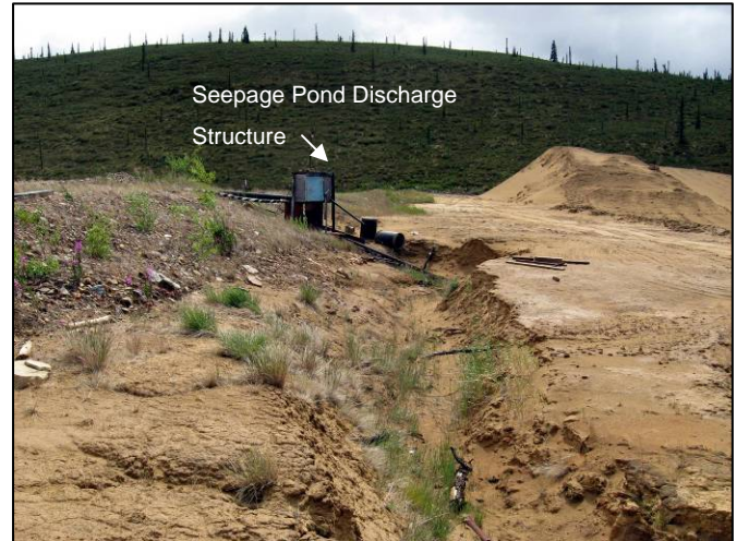
Figure 12 Erosion Gully in Tailings Beach
