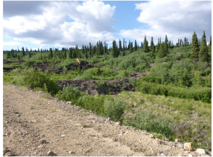
Photo 25. Placer mining activity upstream of H-PC-DSP/WQ-PC-U showing construction of earth dams (June 16, 2015).
