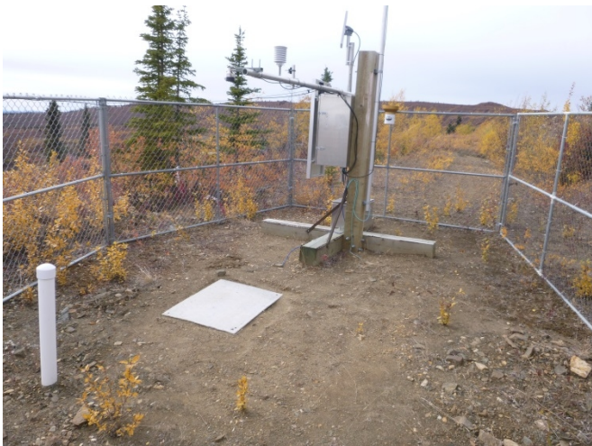
Photo 41. Meteorological station overview.
