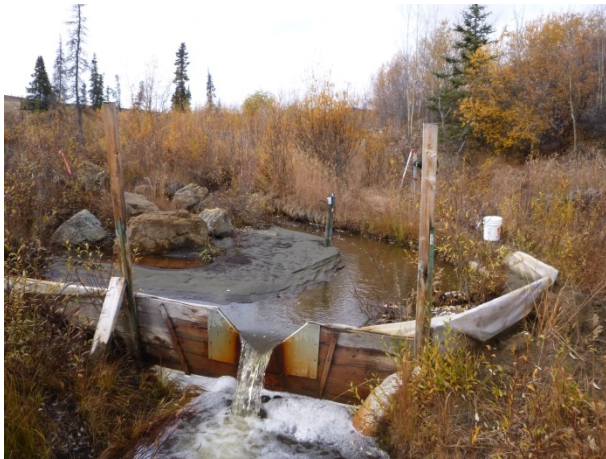
Photo 7. H-DC-M WP – looking upstream showing accumulated sediment.
