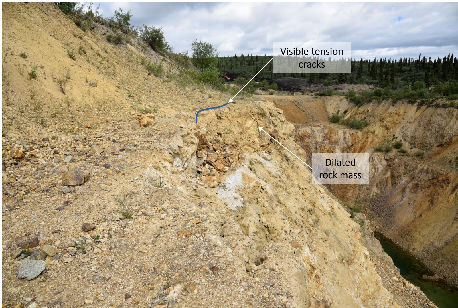
Photo 11: Area above sector 18 showing dilated rock and tension cracks indicating imminent failure. Photo taken June 23, 2016
