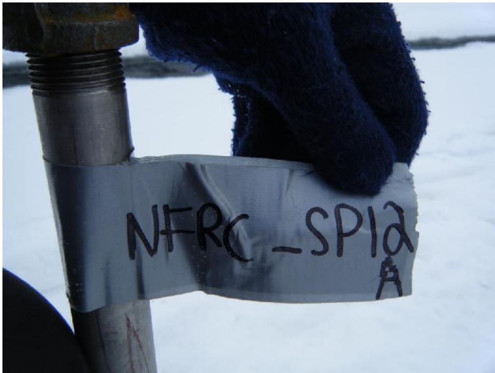
Photo 16. View of label at piezometer CH13-107-PZ012A, November 13, 2013.
