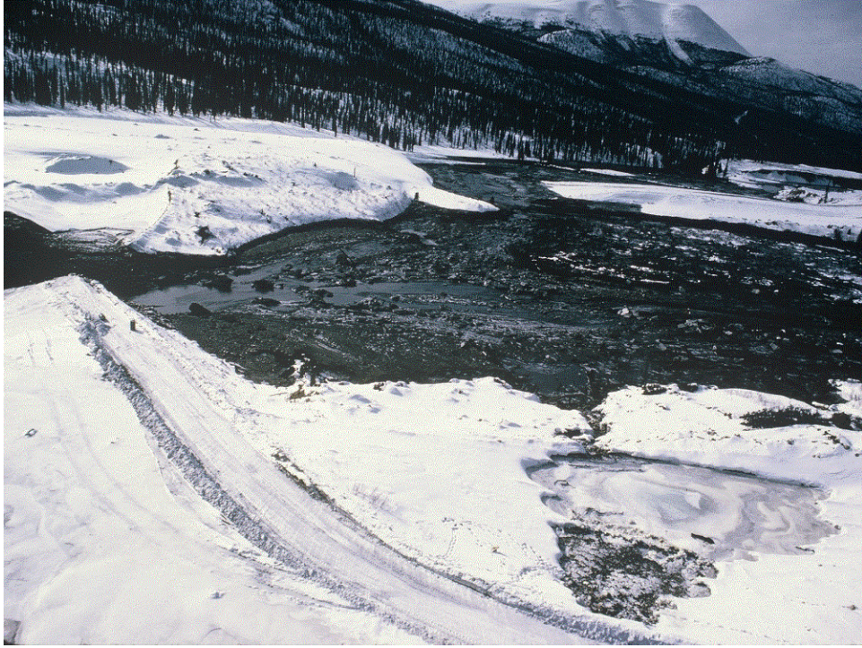
Plate 3. Breach in tailings dam (1975).
