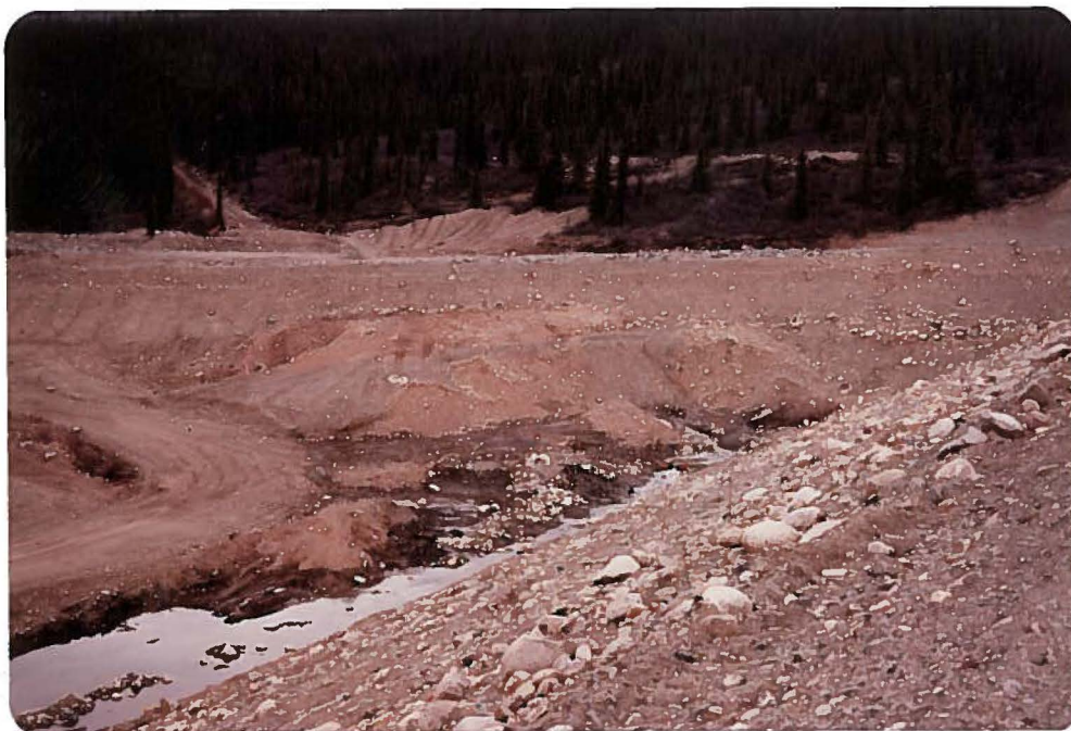
View north showing north abutment area where seepage emerges at downstream toe. Weir No. 1 (Sta 0+215) is near beginning of seepage. (c. 1 June 1982)
