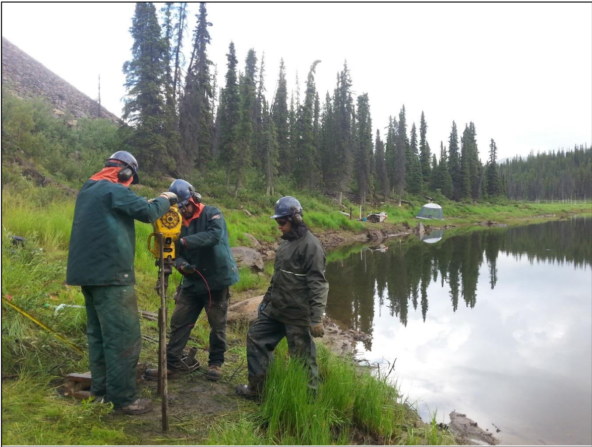
Photo A6: Drillers at MW14-14, advancing a Waterloo profiler tip into the borehole with a Pionjär 140 hammer drill. The Waterloo profiler allowed the team to obtain a water sample from below the depth of refusal.
