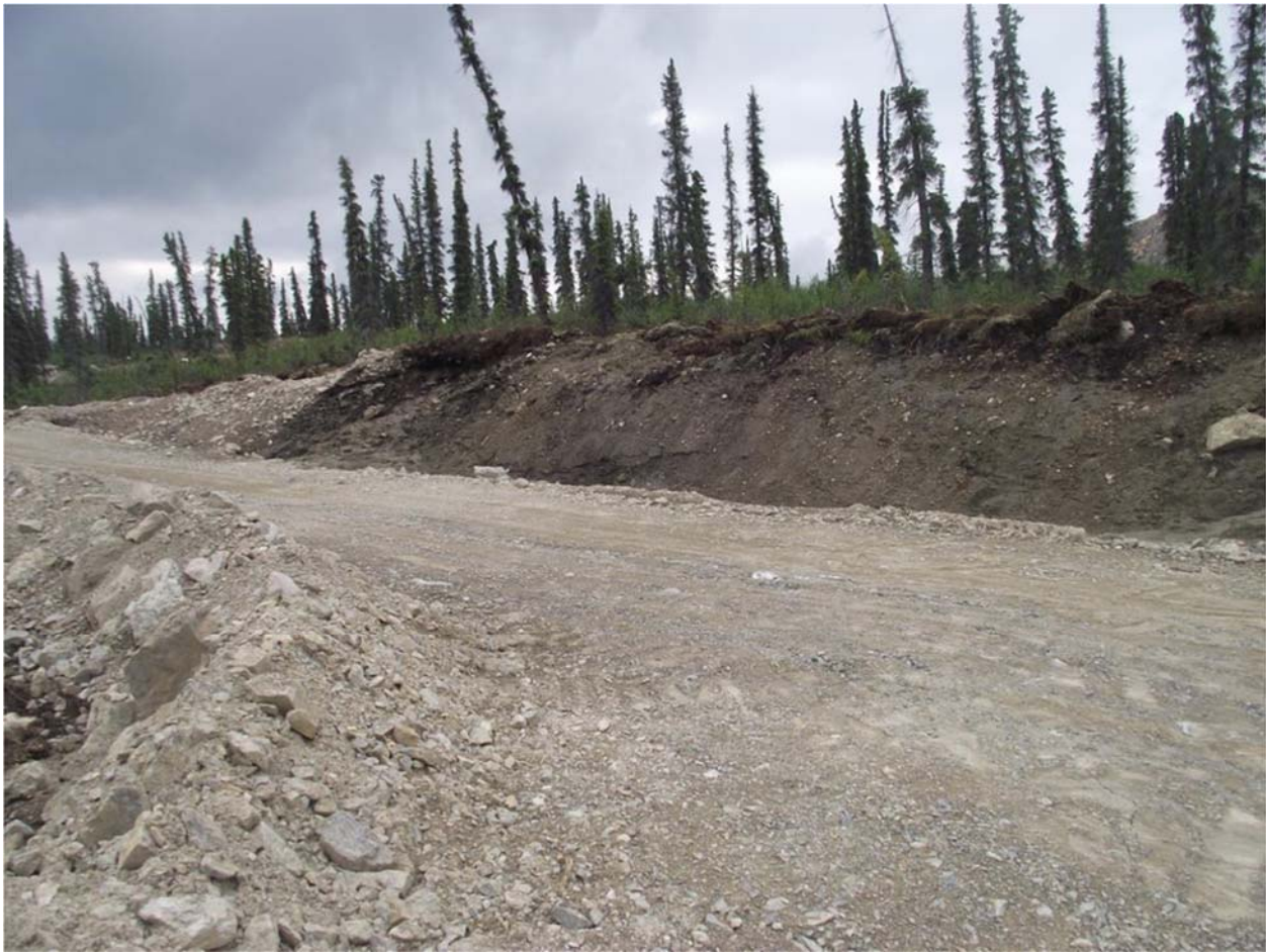
Photograph 5-2 View of lower portion cut slope along access road upstream of NFRD (May 2015). Note thawing and sloughing permafrost immediately to the right of the light coloured rockfill placed on the left side of the cut.
