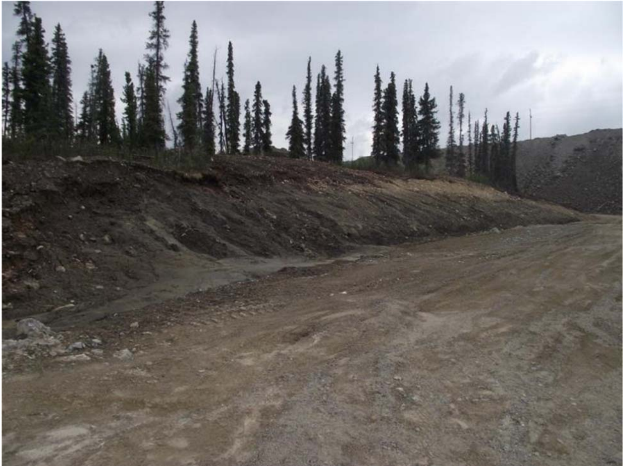
Photograph 5-1 View of upper portion cut slope along access road upstream of NFRD (May 2015). Note thawing and sloughing permafrost of the left side of the cut.
