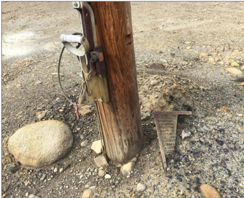
Clearly damaged and non-compliant ground-mat below an overhead 4160V switch. Located nearby the Miller Skid.
