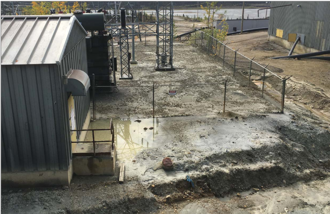
Soil conditions and standing water around the back of the 138kV substation are non-compliant, particularly at the rear entrance to E-Room #1. Given that the front door access is available, an immediate short-term solution is to red-tape and post notices at this entrance on both sides of the rear door.
