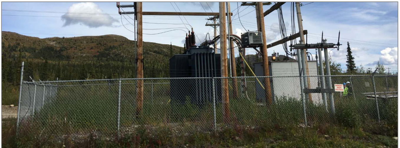
The Van Gorda 69kV step-down station requires vegetation removal and some fresh gravel. The nearby “remote grid” should also have vegetation removal and fresh gravel around the fenceline perimeter.
