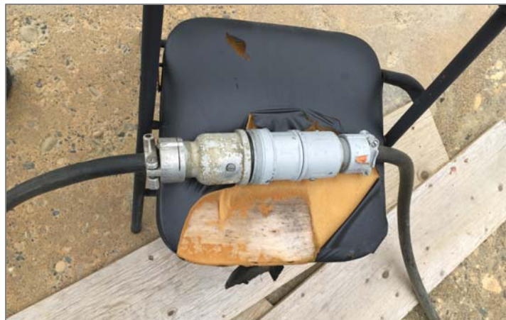
Cable Coupler is missing the Threaded Locking Ring
