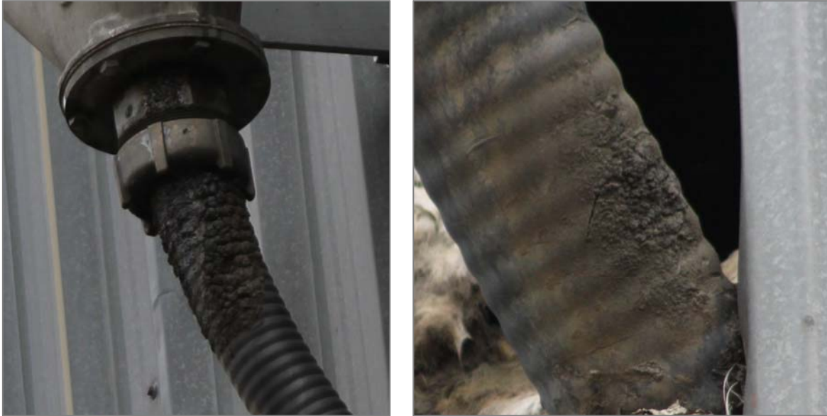
Close-up Photo's of Faulted 4160V Cable Entering the Faro Workshops
