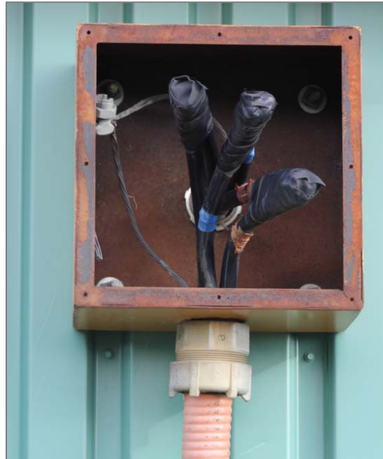
600V Junction box with missing cover at Little Creek electrical room.
