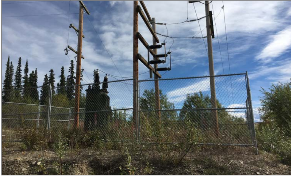
Soil conditions at the 69kV Repeater Station Tap-off are not bad, but vegetation removal is recommended.
