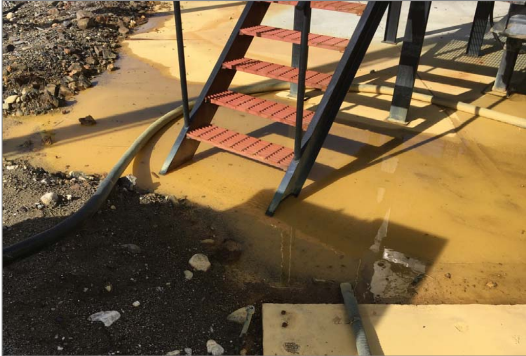
... but the grid and gravel do not extend around the 600V generator that is electrically tied to the HV transformer. Shown here, the access steps and handrails to the generator enclosure are in standing water and do not appear to be directly bonded to the station ground.
