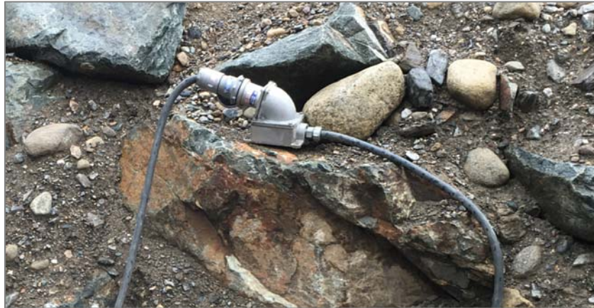
Wall-mount Receptacle being used as an Extension Cord End at the Filter Station near the Int. Pond
