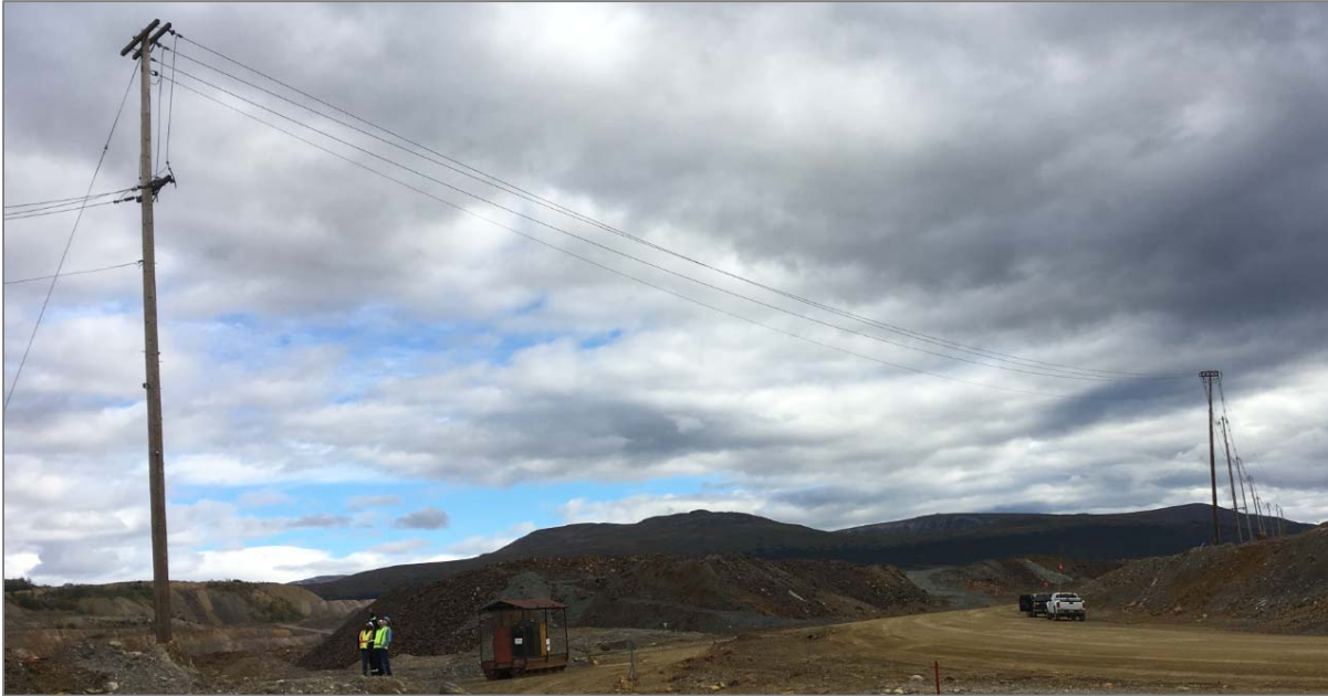
This long 4160V span near the Faro Pit has insufficient phase to phase clearances, at high risk of flashover during high winds and inclement weather.
