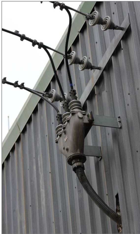
Faulted 4160V Cable Entering the Faro Workshops
