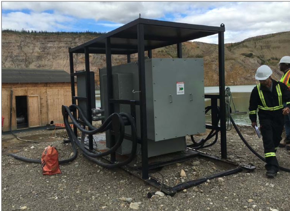
4-Rod ground-grid and clean gravel spread at the 4160V Faro Pit pump station are done well.
