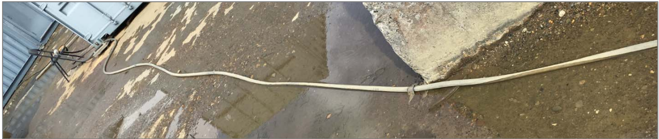
IWTP: Temporary (>1 week) Power Cable Routed Through Pedestrian Area in Standing Water
