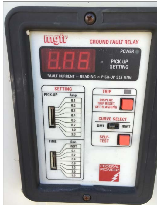
Ground Fault Relay at Groucho Pond is Out of Service
