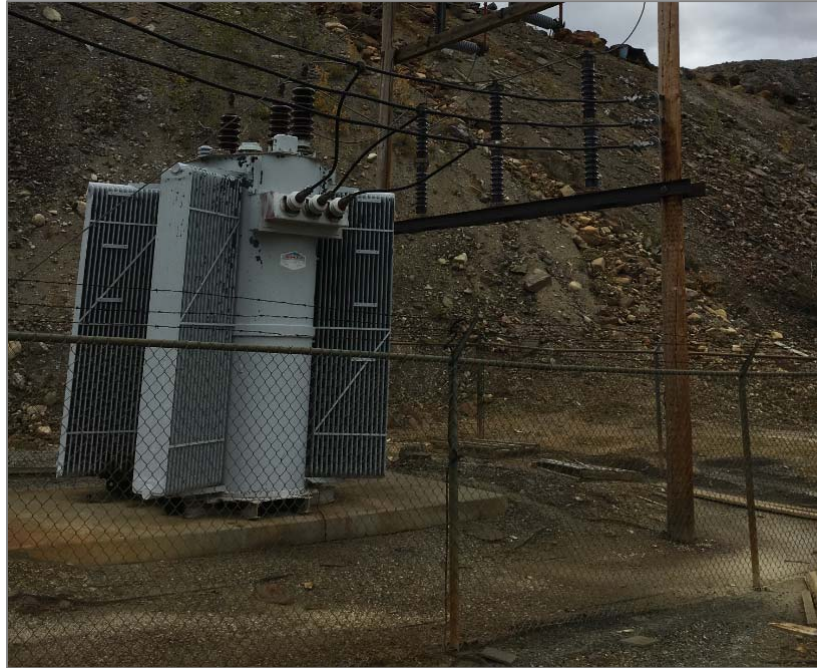
The 69kV Step-Up Station requires a fresh layer of insulating gravel for code compliance.
