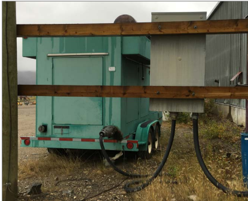
Backup Generator at the Norcan Shop uses a mining coupler without adequate ground-fault / ground-check protection. At 600V it presents a lower risk but is still non-compliant.
