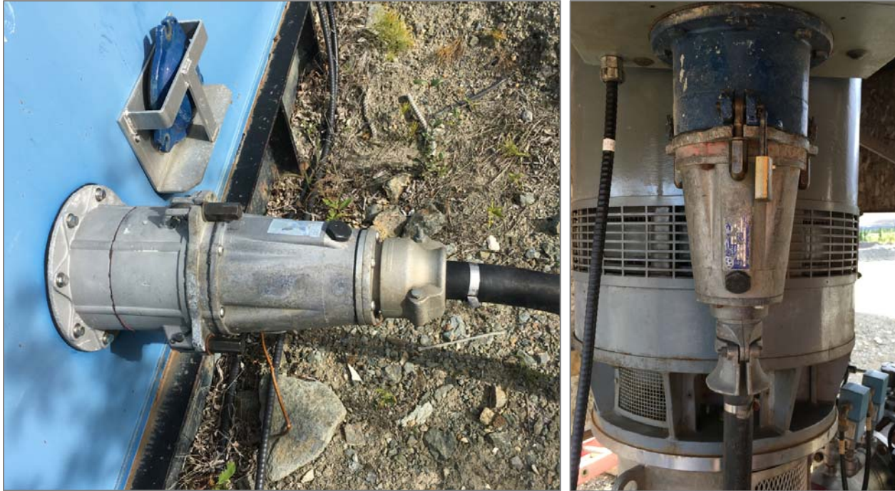
Outgoing 4160V connectors to the Van Gorda pumps are also non-compliant, as the upstream ground-fault / ground-check relays are out of service.
