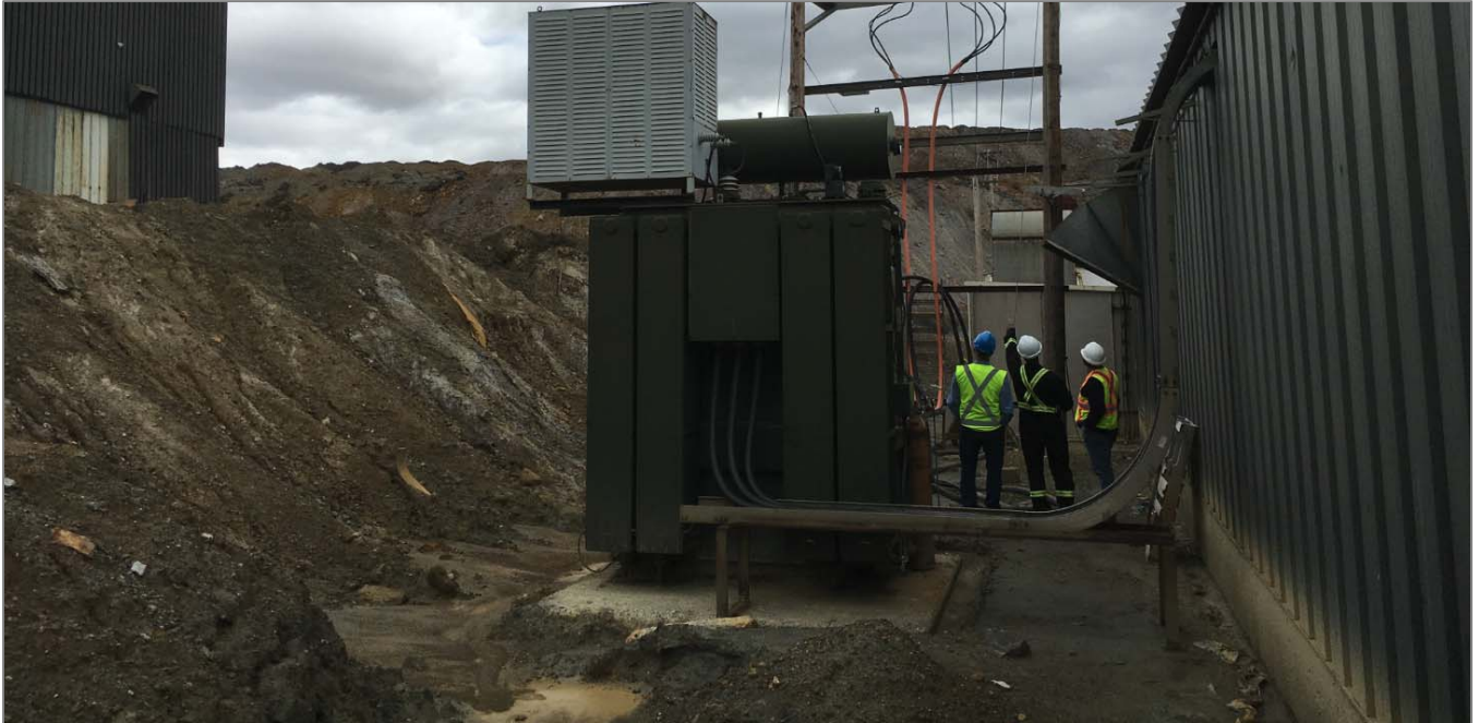
Soil conditions around the T3 isolation transformer are non-compliant. Recommended solution is simply to remove T3 from service as soon as practical.
