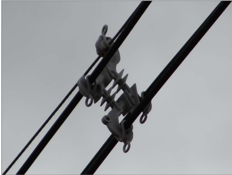
Bundled Multiphase Insulators used for 7 spans of Line near Faro Pit are Notoriously Unreliable
