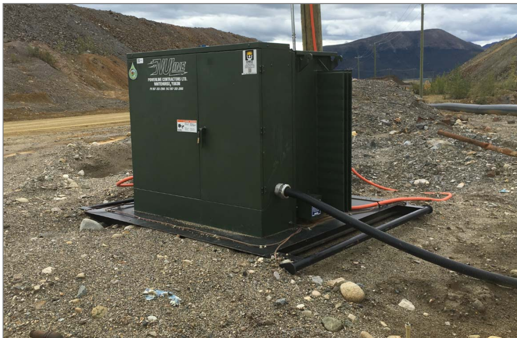
The 4160V step-up transformer at the Faro Pit standby generator appears to be compliant with a 4-rod grounding grid and a layer of relatively clean gravel spread around it...
