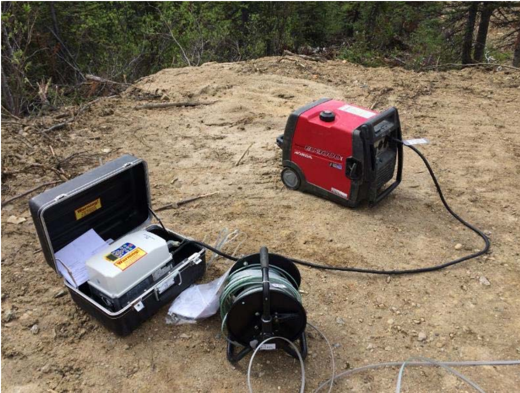
Photo 2. Pump Controller, generator and pump power line at CH15-106-MW007
