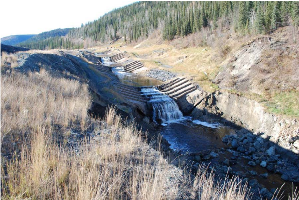
Photo #8: Further upstream, undercutting has occurred at the fourth gabion structure leaving the lower portion of the baskets hanging. Photo taken on September 21, 2010.
