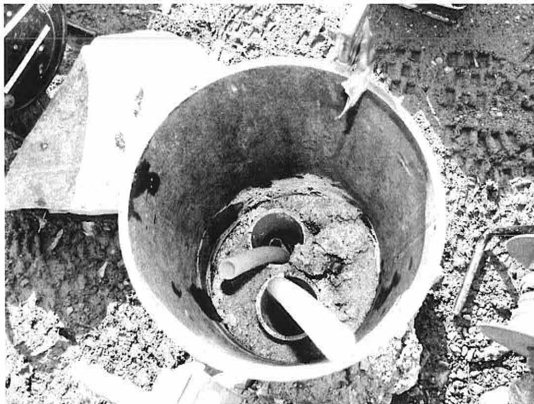
Inside P2001A and B – silica sand and bentonite inside the annular space has been pushed up to above the top of pipe, May 31, 2009.
