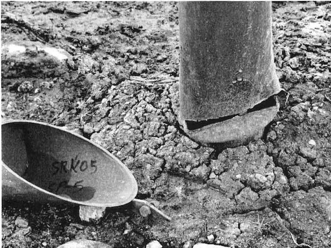
The casing and well of SRK05-SP5 had been damaged prior to May 30 th , 2009.
