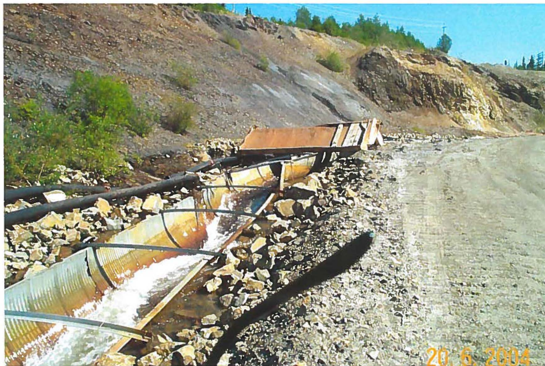
Photo 32: Section of flume that experienced most severe lifting during flood.
