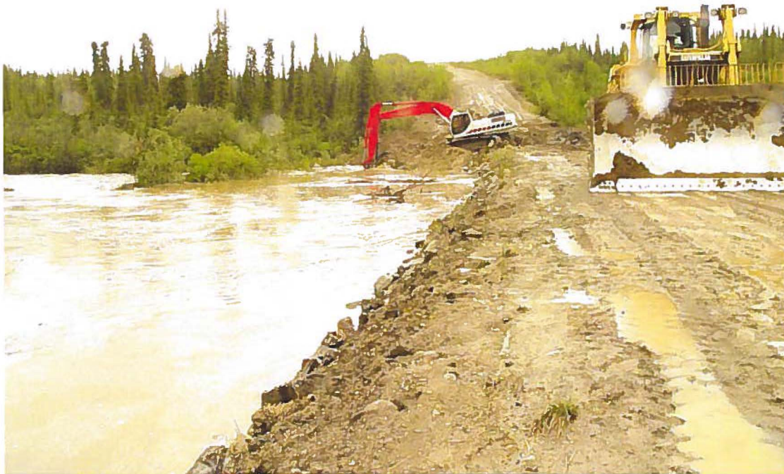
Photo 15: Ponded water upstream of Headworks embankment (June 8, 2004).
