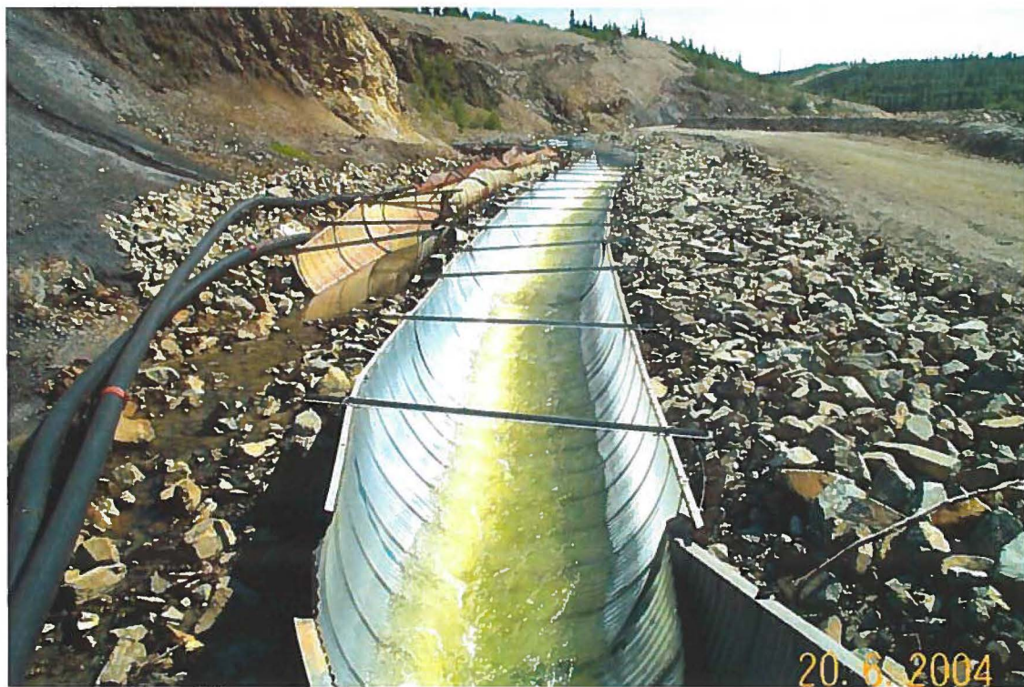
Photo 34: View upstream of recently installed flume section. Original flume section shown to the left of new flume.
