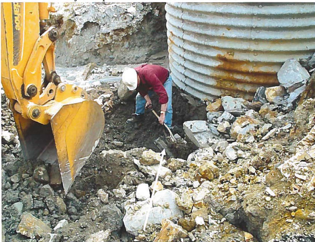
Photo 22: Exposed crown of separated joint in 2000mm Ø culvert.
