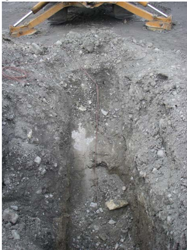
Photo 22: Matric Suction Sensors installed in the Test Pit on L#2
