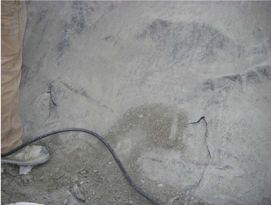
Photo 13: Tears in the Liner of L#2
