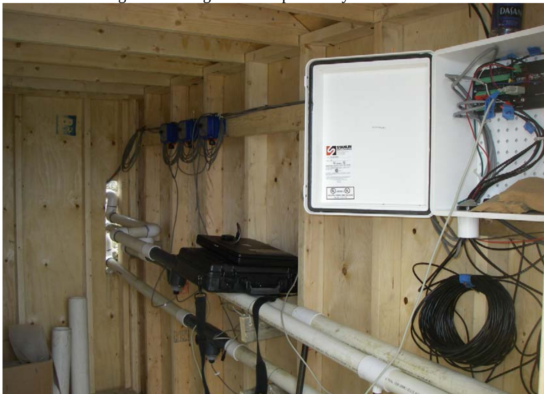
Photo 28: Detail of the Instrument Hut with the CR1000 Data Logger Housing Box in the foreground and the Flow Meter data loggers in the background
