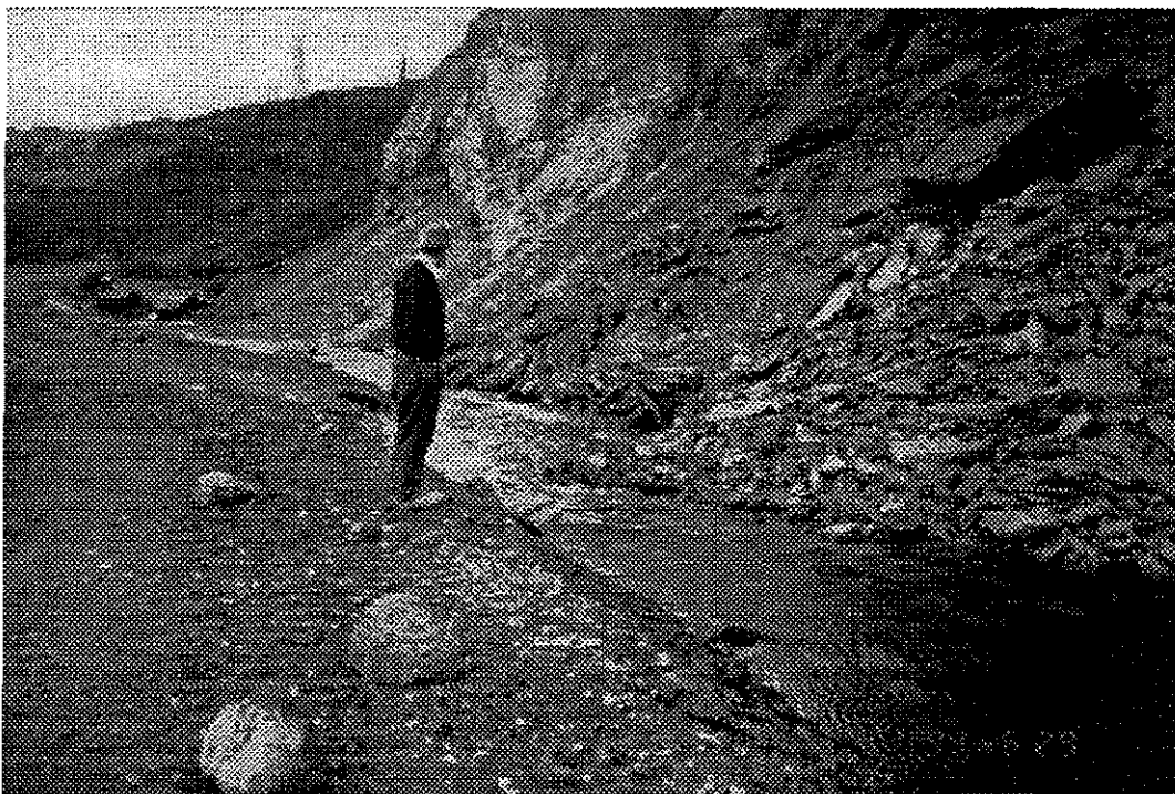
Photo #1B, initial condition of flume following wall failure
