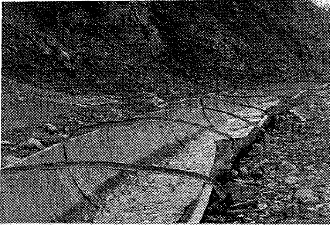
Photo #7a, damaged sections approx. 4+95 to 5+35
