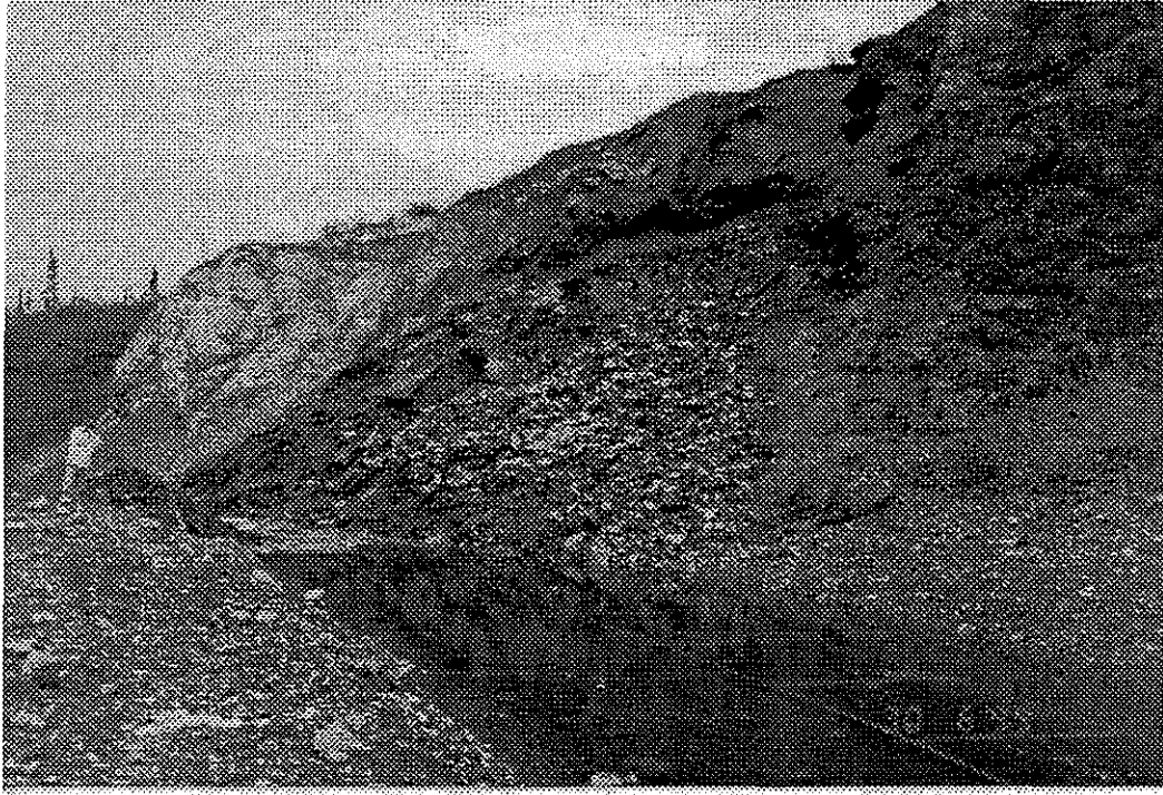
Photo #1A, initial condition of flume following wall failure
