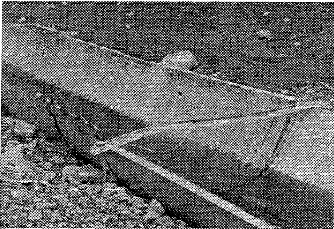
Photo #7b, improperly installed patch at approx. 5+17
