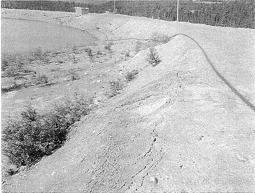
Photo11 Bank Erosion on east approach road
