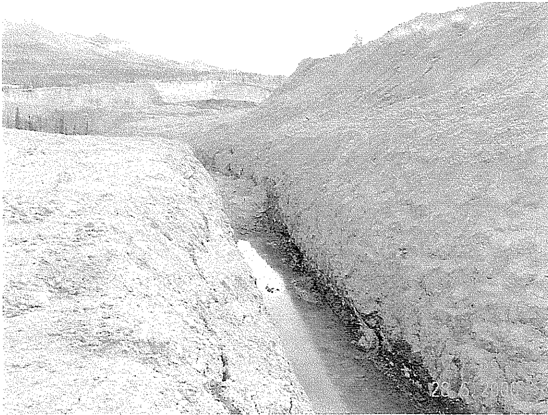
Photo 9 Poned Water in the diversion ditch
