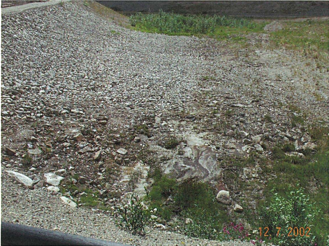
Photo 25: Seepage zone at the north toe of the sludge dyke.
