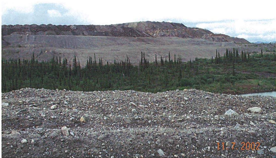
Photo 2: View looking south of the resloped area of the till starter dyke
