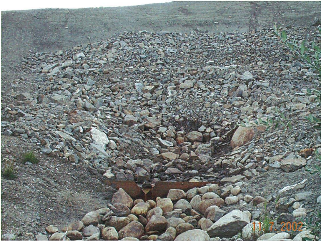
Photo 5 : Drain #6 at toe of the starter Dyke on North side of Vangorda Waste Dump
