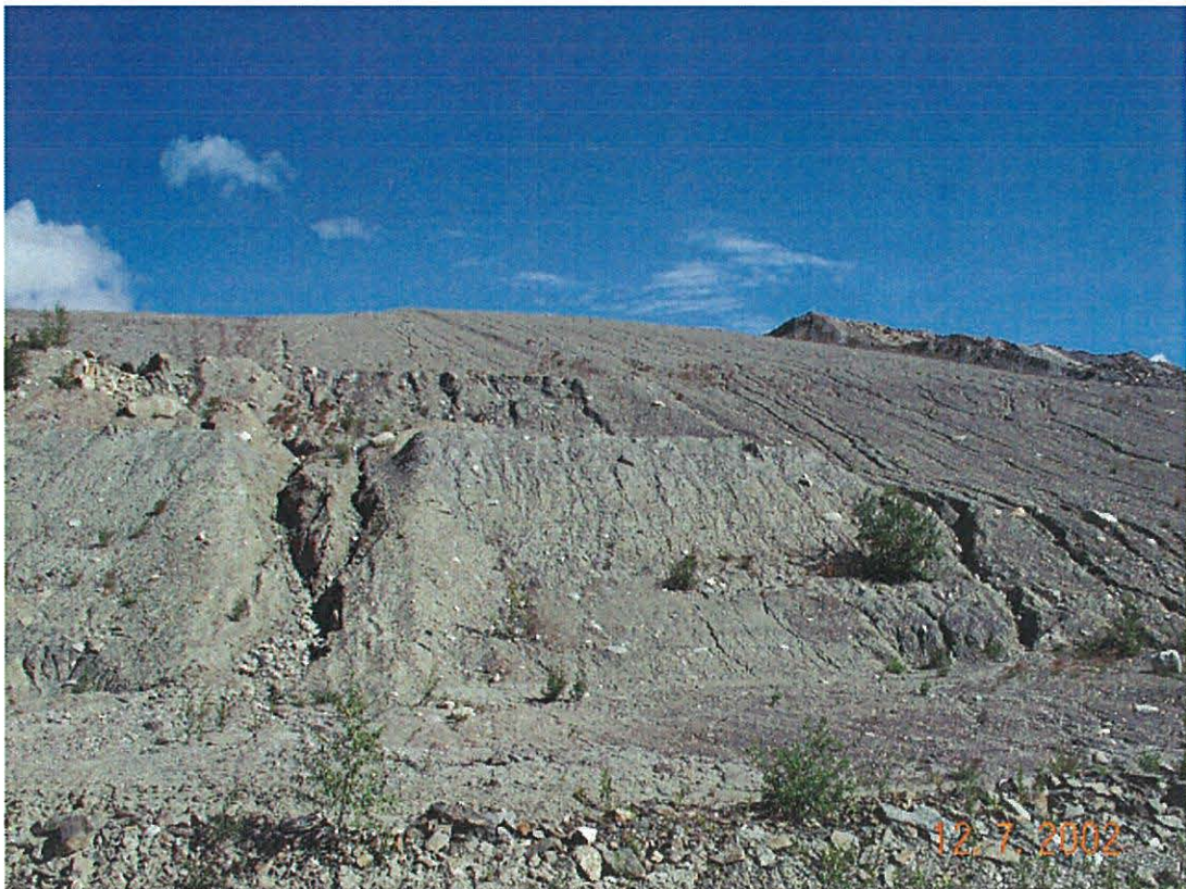
Photo 12: Erosion gullies at toe of till cover on south side of the Vangorda Dump
