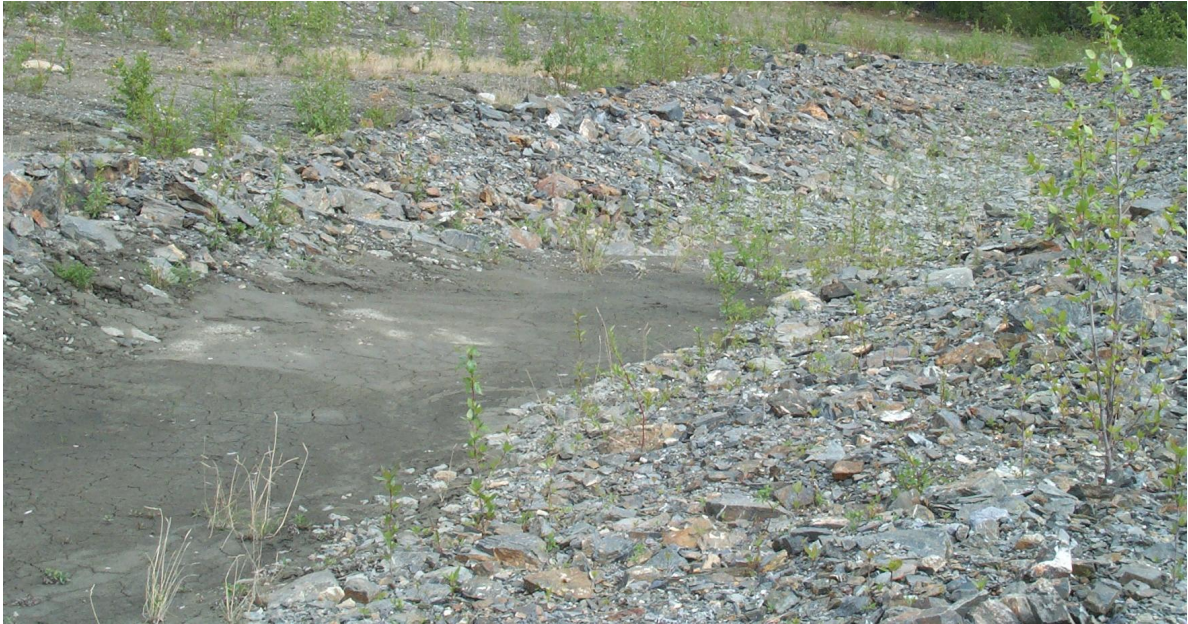
Photo 4: View of the collection drain at the toe of the till cover. Note the accumulated fines that have been washed off the slope.
