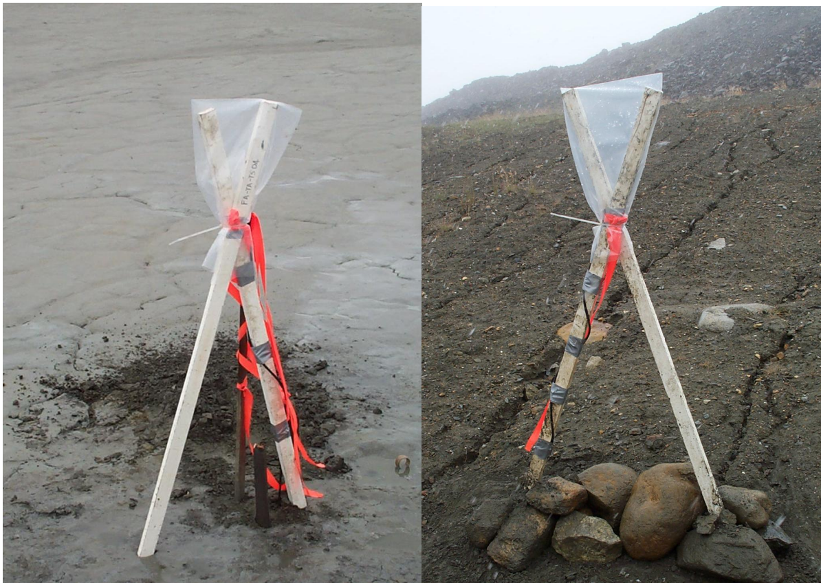
Photo 20: Examples of the thermistor installations on (1) Rose Creek tailings and (2) Vangorda waste rock pile starter dyke till.
