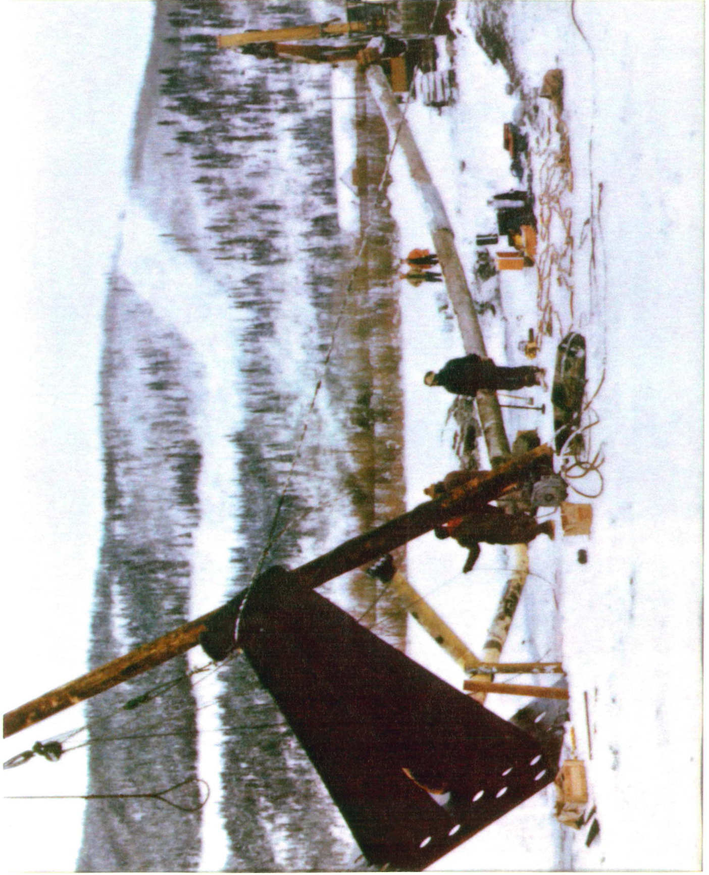
SEWAGE OUTFALL - Dawson City
