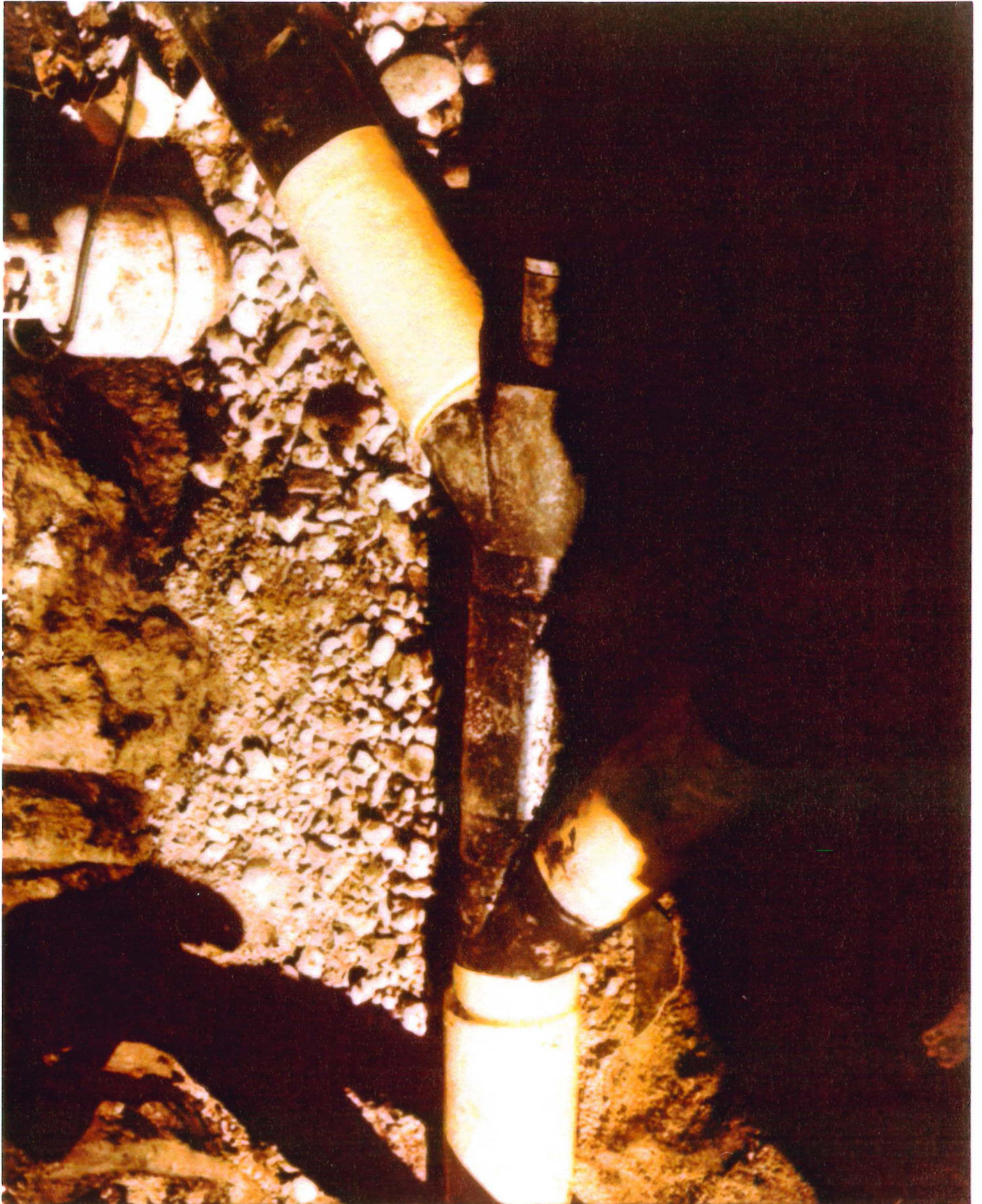
SEWER HOUSE CONNECTION – Dawson City
