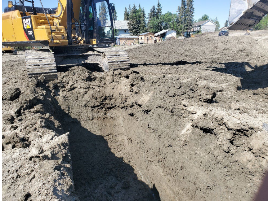
Photo 2: TP04 showing unconsolidated soil condition.
