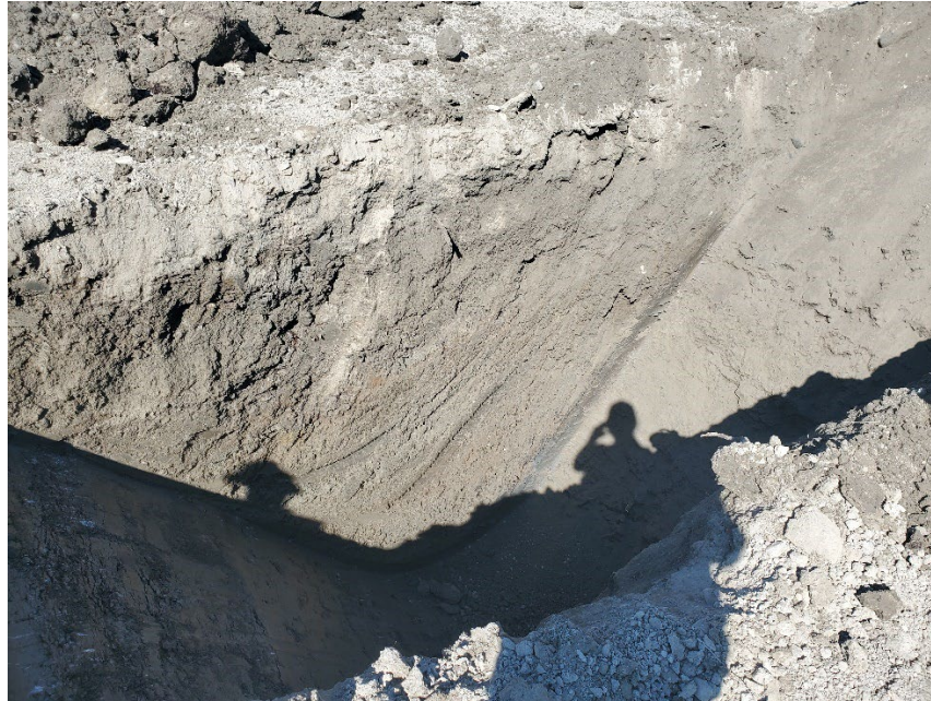
Photo 4: TP02 profile shows increased consolidation at depth of approximately 1.0m
