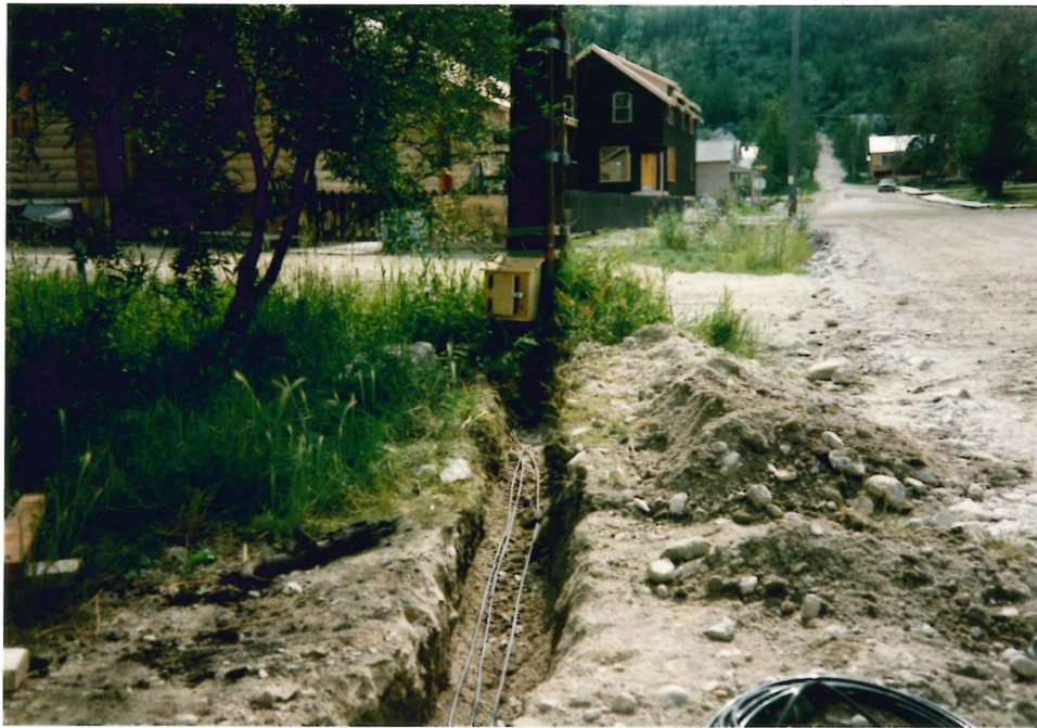
PLATE 3 : General view of thermistor cable leads and read-out box (Church St, 1985-07-05).
