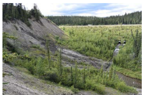
Slope failure by McIntyre Creek
