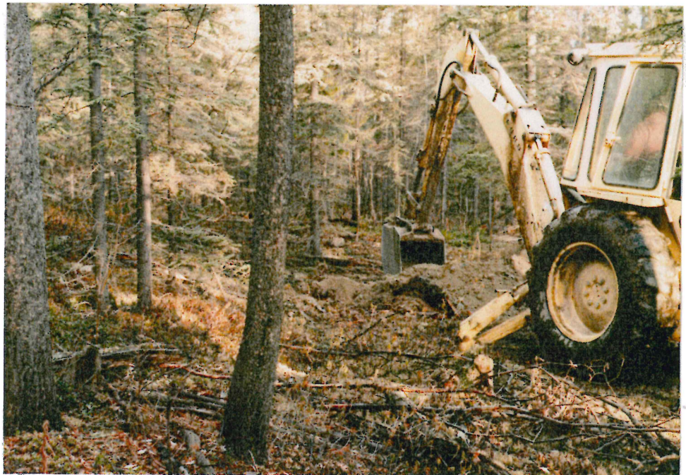
#1-18 LOOKING NORTH-WEST @ TP 86-G SITE. EXIST TRAIL (ACCESS ROAD) IS TO RIGHT OF BACKHOE.
