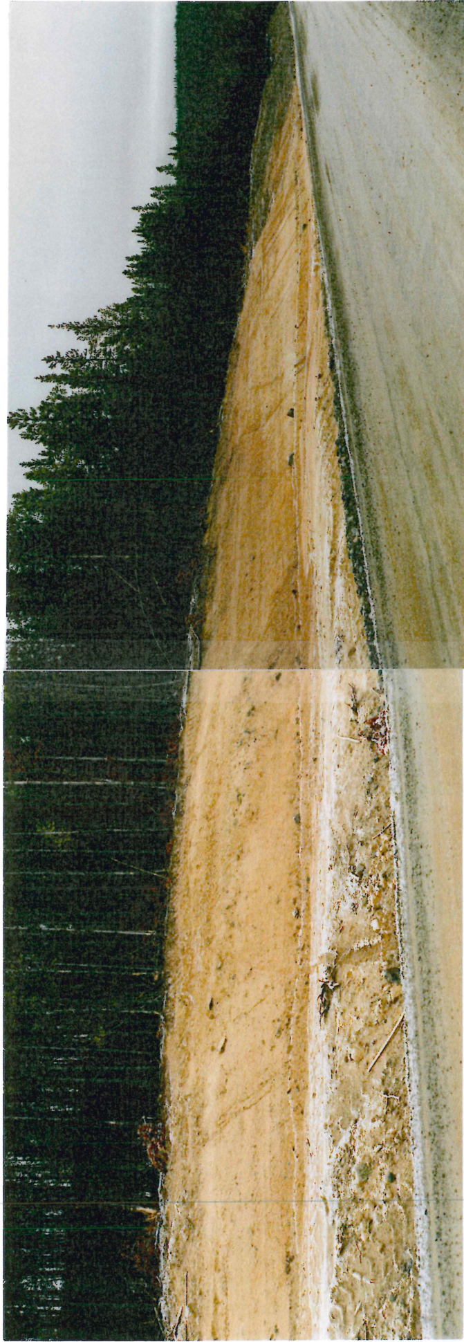
# 2-20, 2-21 CUT SLOPE ALONG QUARRY ROAD BROWN FINE TO COARSE SAND, SILTY (DECOMPOSED GRANITE)
