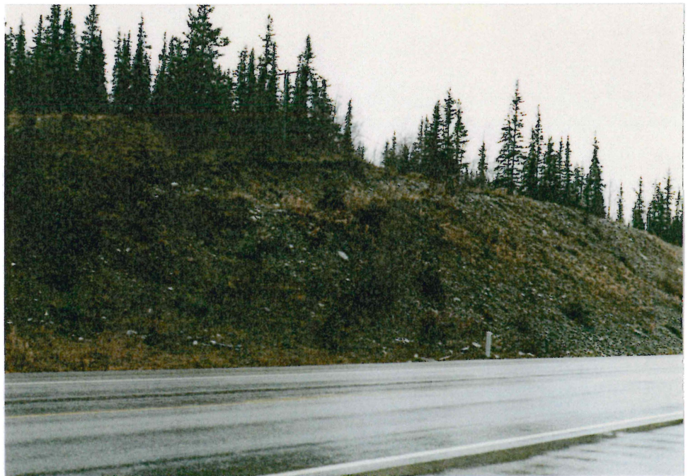
# 3-37 SAND & GRAVEL EXPOSURES ON WEST SIDE OF ALASKA HIGHWAY ON SLOPE BELOW TP 86-23 & 86-24
