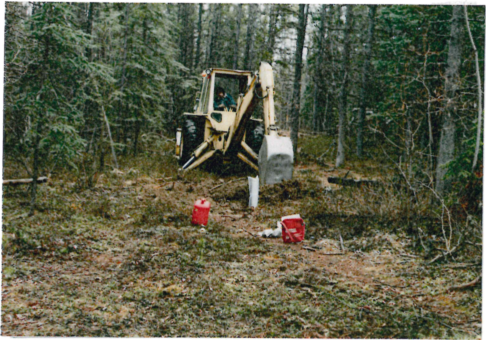
# 4-24 LOOKING SOUTH-EAST ALONG EXIST. CUT LINE TO TP BG-31. NOTE 4" PVC PIPE INSTALLED IN PIT PRIOR TO BACKFILLING, FOR PERCOLATION TESTING
