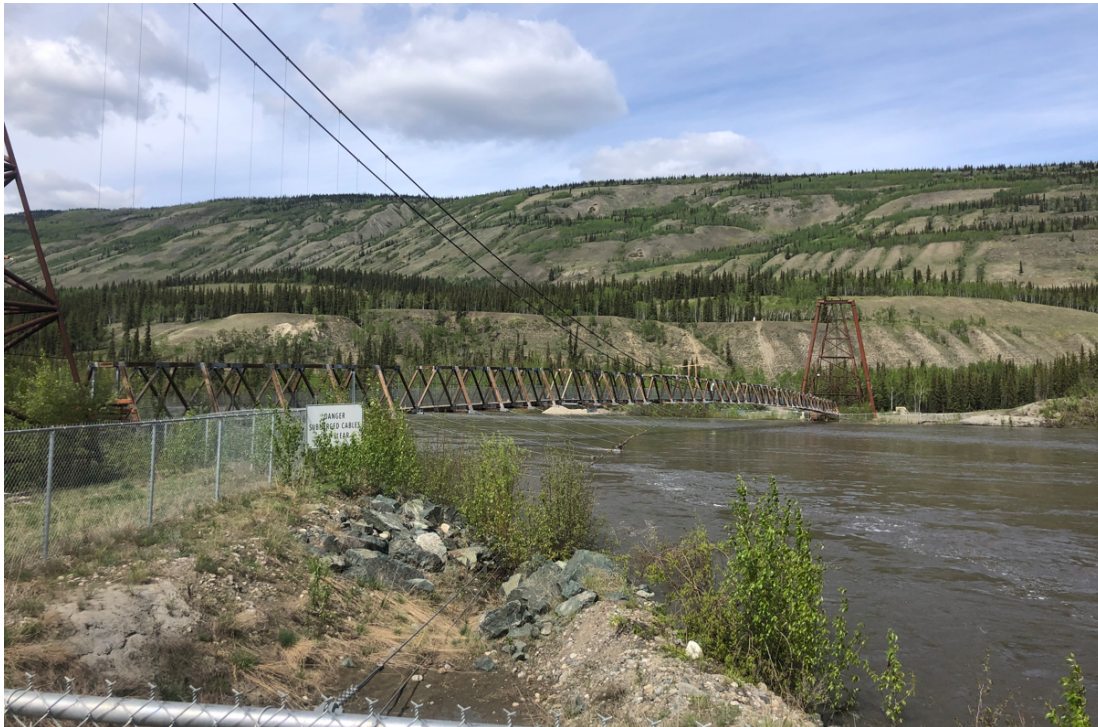
Photograph 1 Ross River Pedestrian Bridge During 2022 Flood (June 7, 2022)
