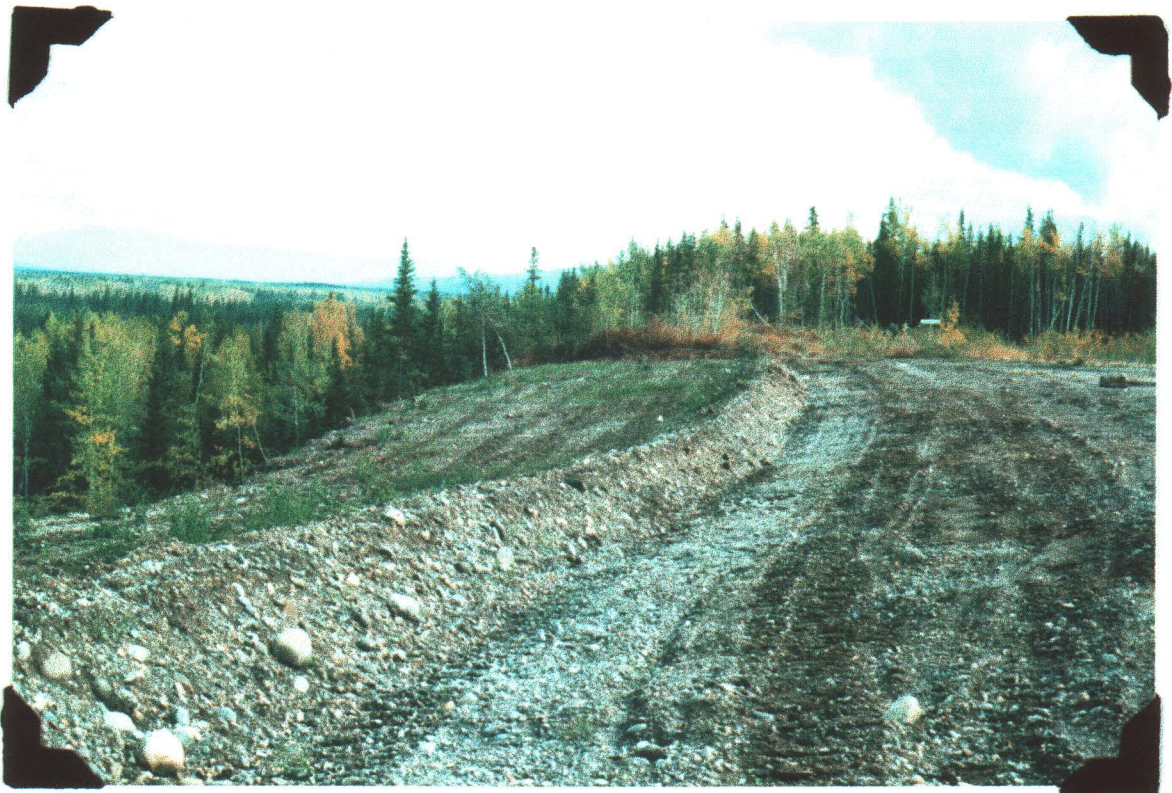
Figure 6. Mayo Landfill - Dump crest with recent fill cover.
