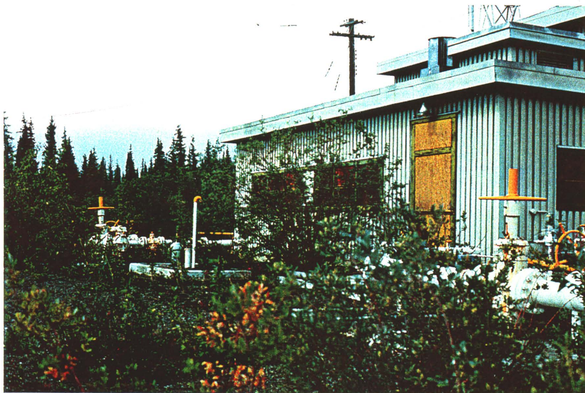
Photo 17: Pump building at Donjek. Various associated valves along the pipeline are in the foreground.
