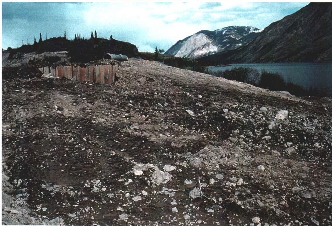
Photo 21: Depressions at South Wall requiring Additional Material
