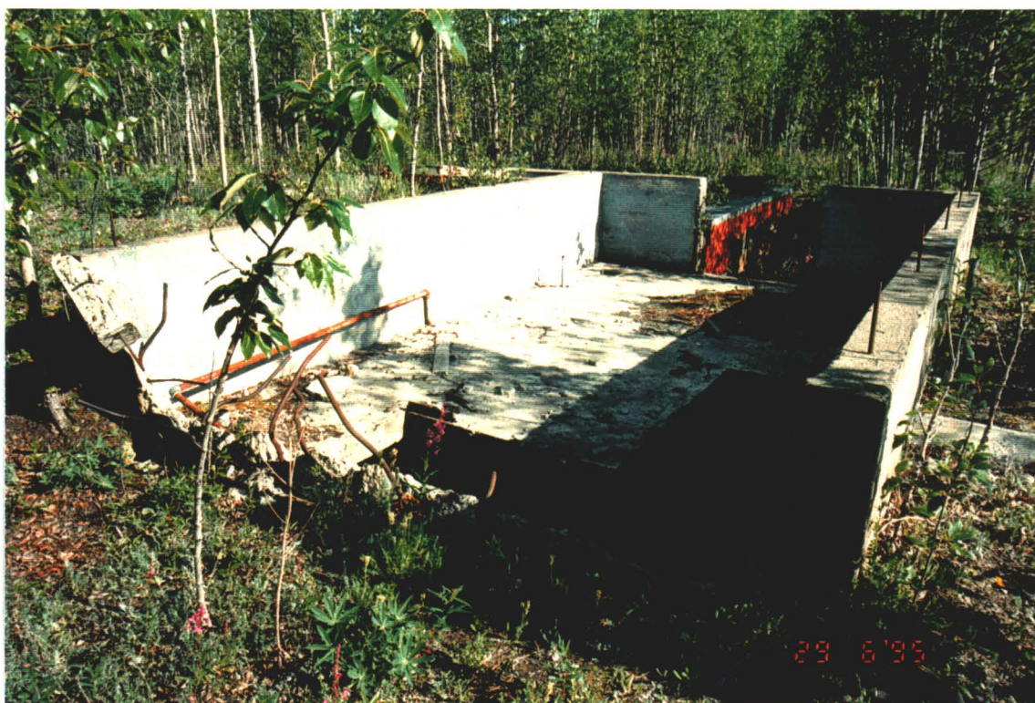
Photograph III-21: The pump house foundation as viewed from the southwest with the opening to its basement visible.
