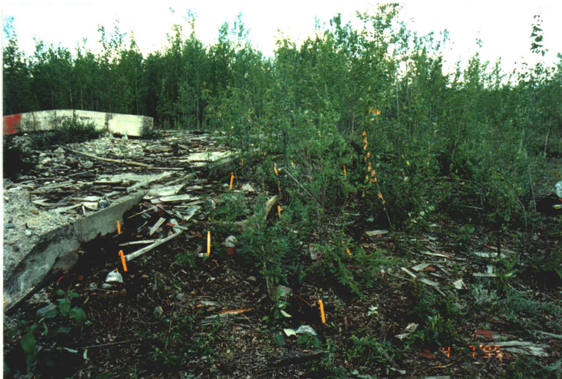
Photograph III-23: Pegs indicating the delineation of contamination on the eastern side of the powerhouse foundation (sample series SN33).
