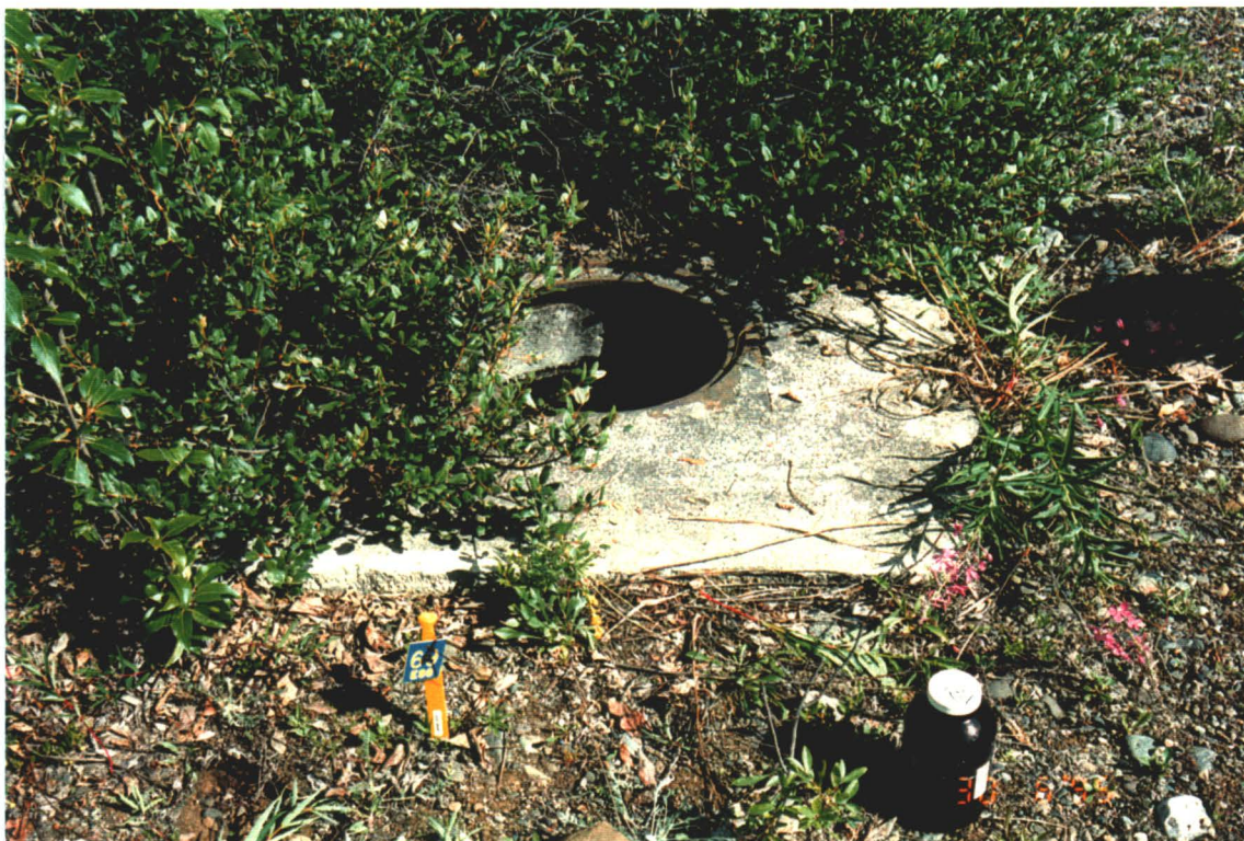
Photograph III-31: Debris collected from the bottom of this manhole (O6104) contained concentrations of copper and zinc which exceeded the criteria.
