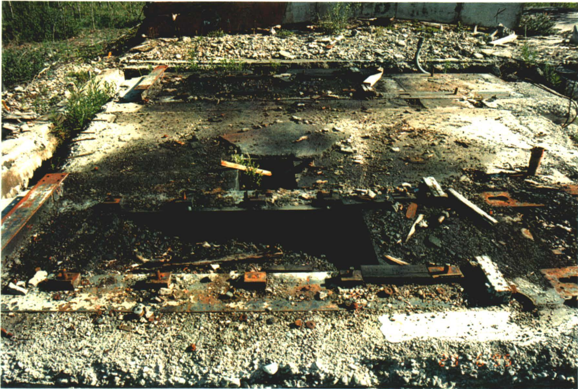
Photograph III-22: Oily sludge on the powerhouse foundation contained PCBs at concentrations exceeding the level regulated by CEPA.
