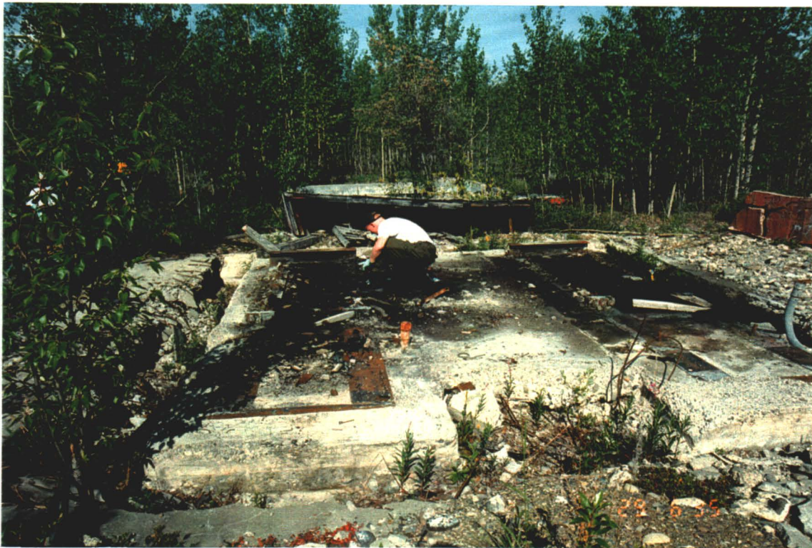
Photograph III-19: The oil-stained south half of the powerhouse foundation as viewed from the east.
