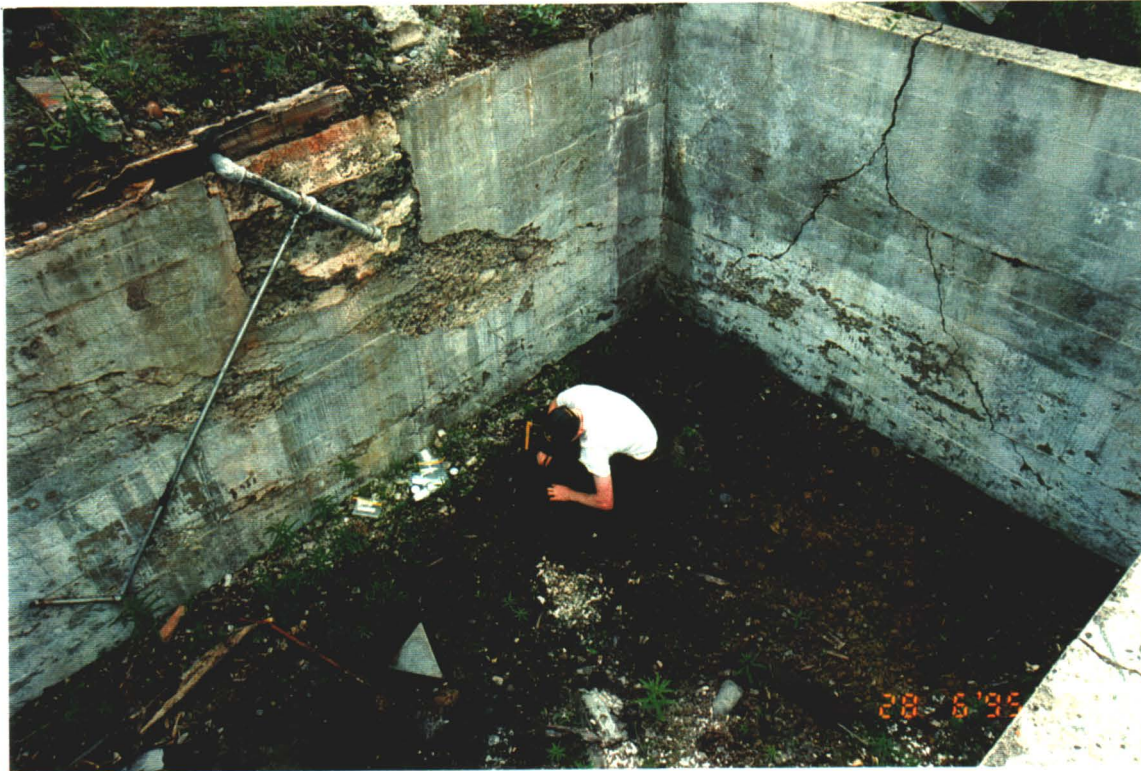
Photograph III-10: PCB concentrations in violation of CEPA and high levels of dioxins were found in soils collected in the barracks basement (G6119A/B).
