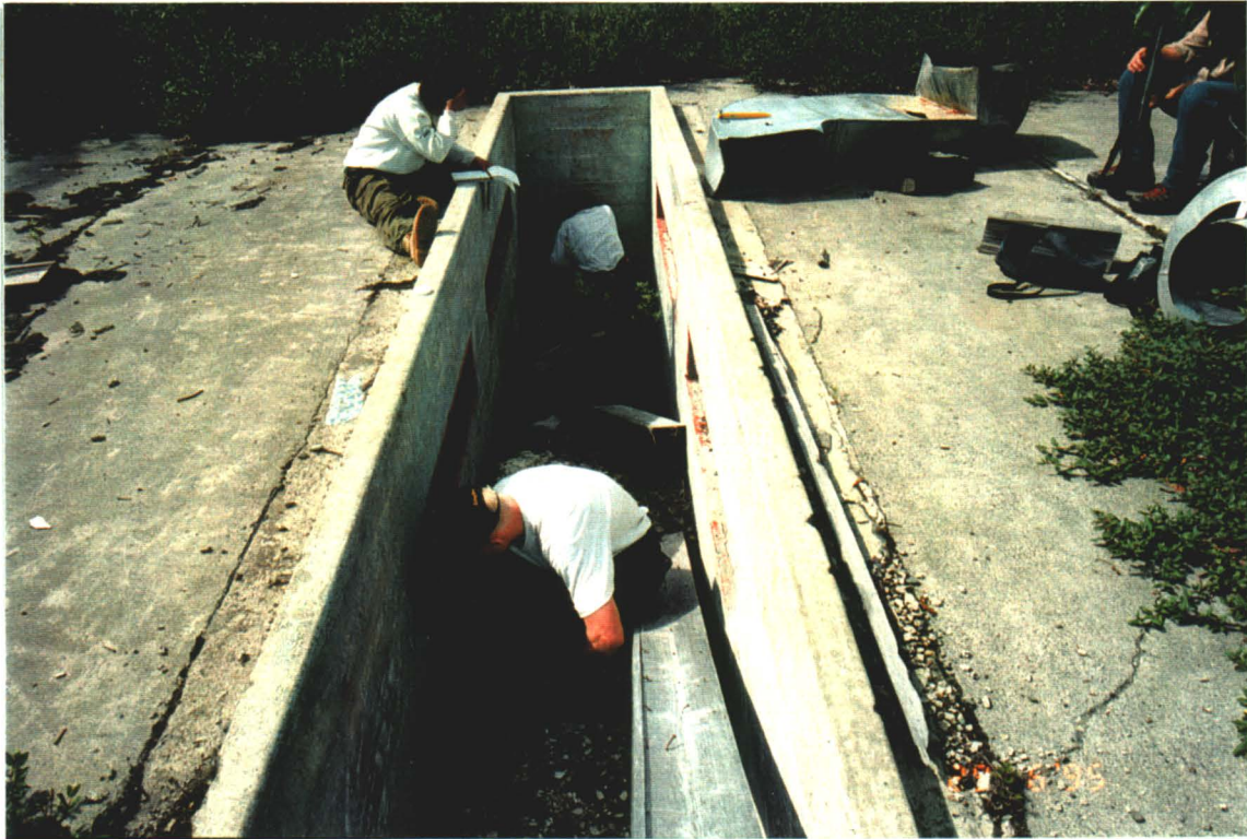
Photograph III-27: Debris from the larger oil-change pit at the garage (G6153) contained high levels of PCBs, dioxins, pesticides, PAHs and inorganic elements.
