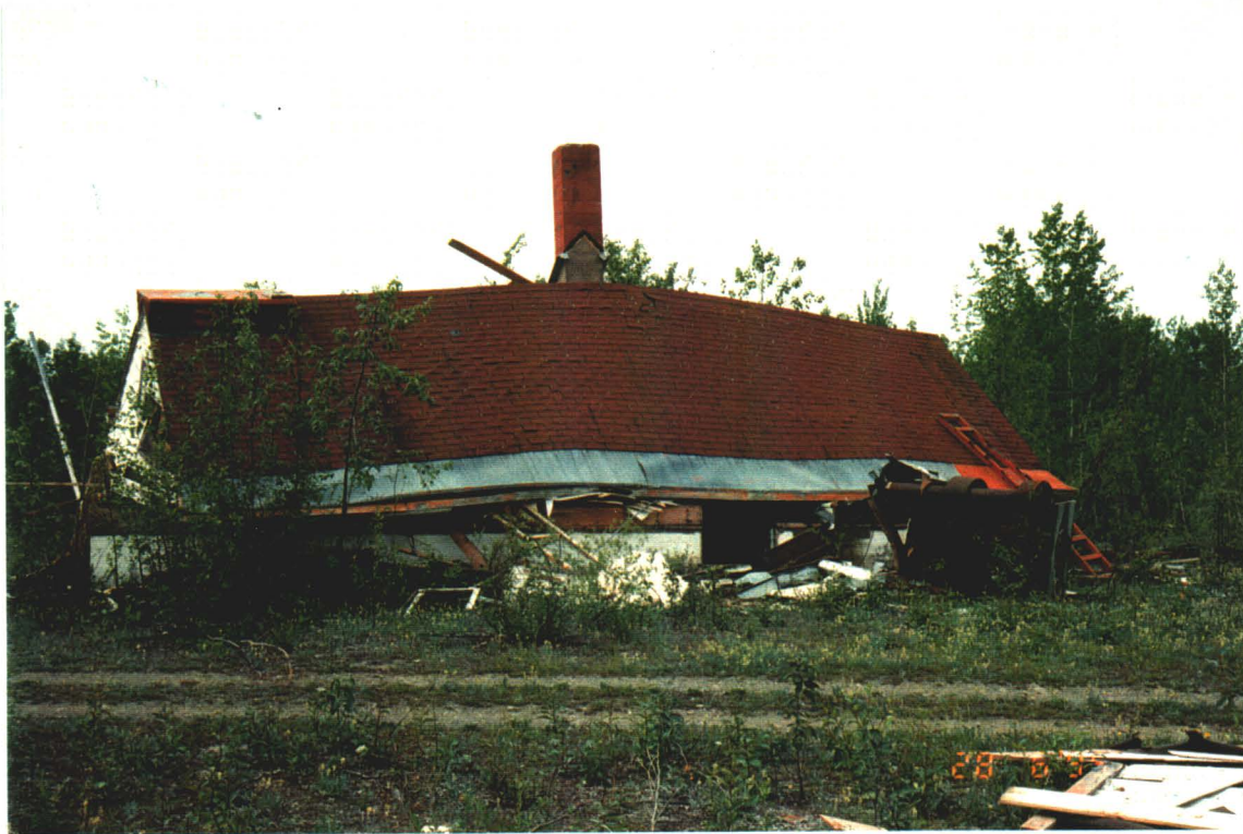
Photograph III-3: View from the south of the tower building in 1995 following its partial demolition.
