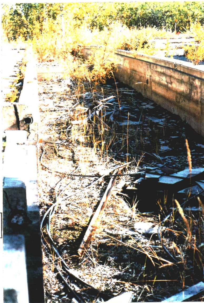
Photograph 30-P6: Channel on the north side of the concrete foundation. Note small pit in the right foreground.
