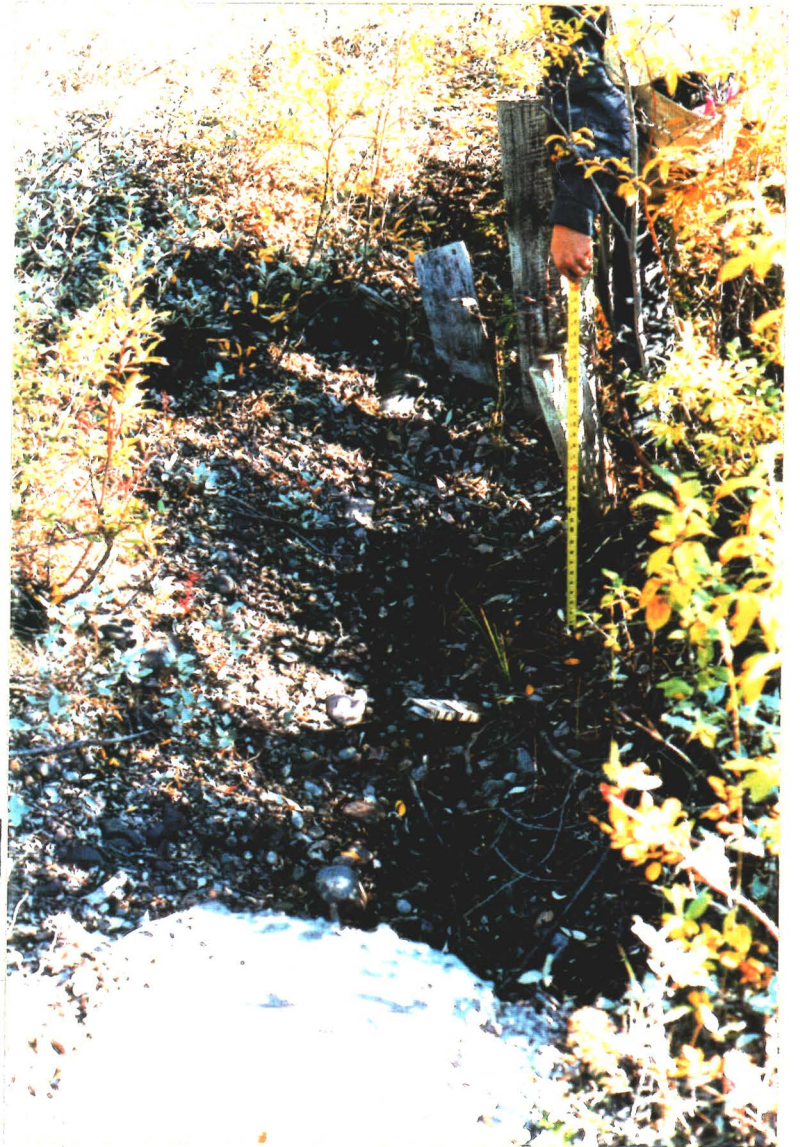
Photograph 30-P8: Depression on the outside of the northwest corner of the concrete foundation.
