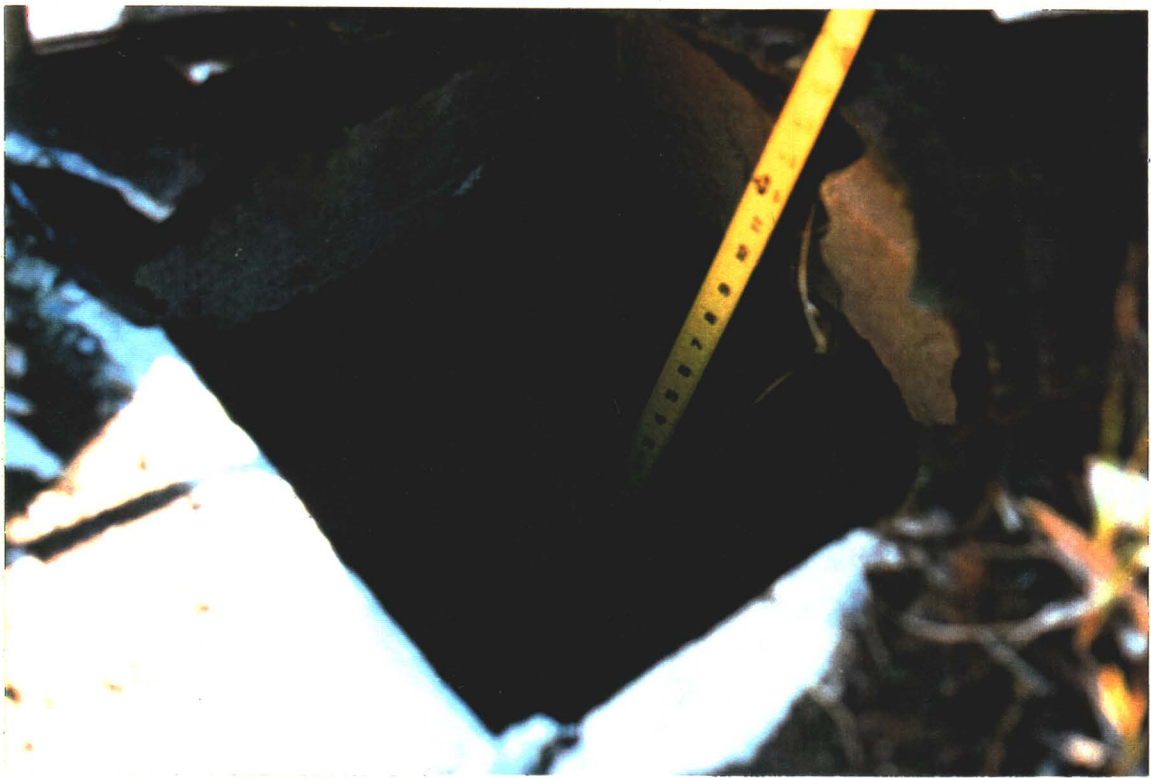
Photograph 30-P7: Small pit in the channel of the concrete foundation.
