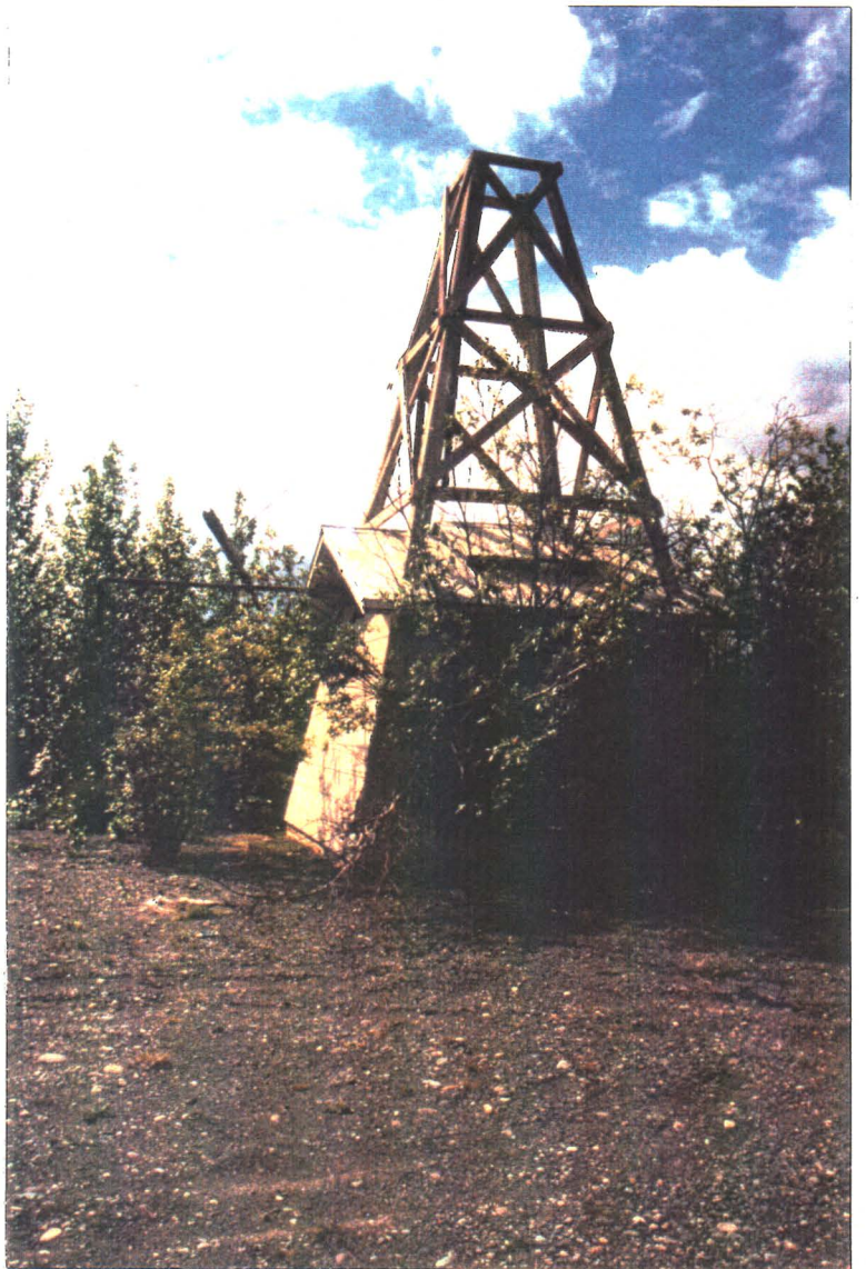
Photograph 30-P1: South facing view of pumphouse. Gravel access road is in the foreground.
