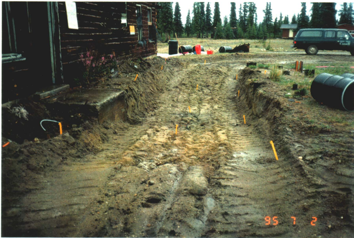
Photograph III-5: Excavated area at AA108 and AA115, the powerhouse south stain after removal of DCC-I contaminated soil.
