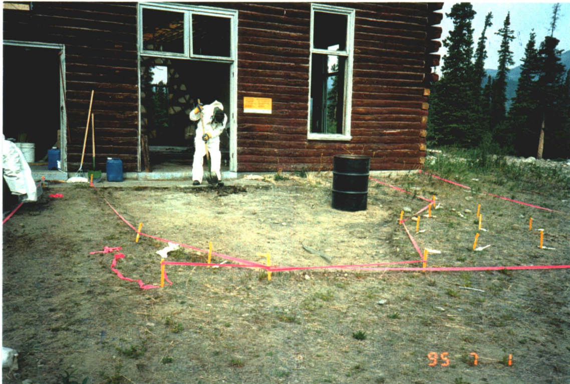
Photograph III-2: Excavation and barrel containment of DCC-II/CCME R/P PCB-contaminated soils at AA101, the powerhouse east stain.
