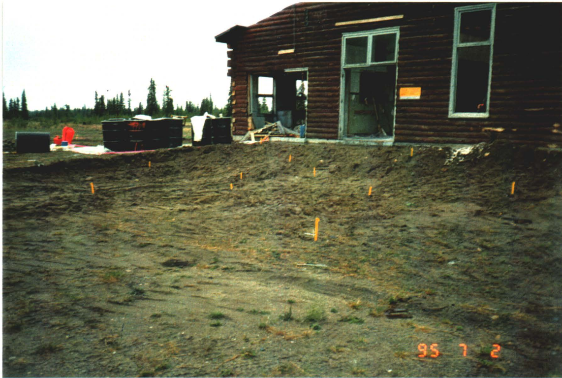
Photograph III-3: Excavated area at AA101, the powerhouse east stain, after removal of DCC-I contaminated soil.
